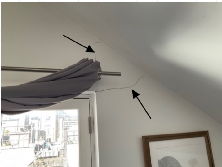
Cracking in 1st floor front bedroom
