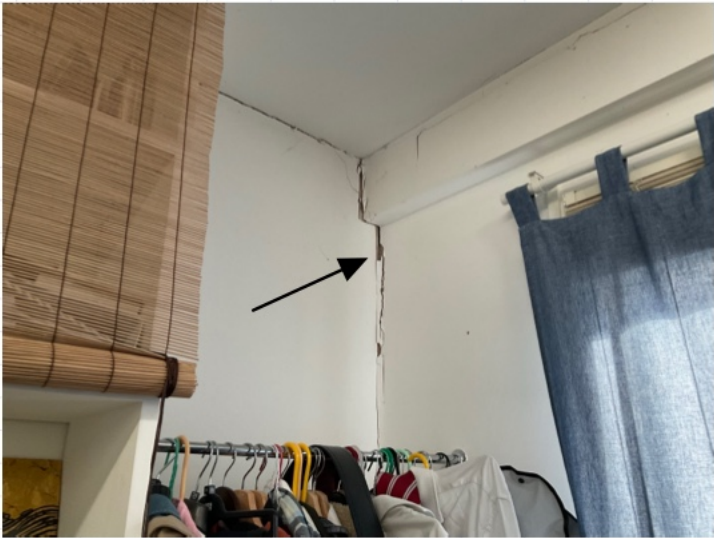
Cracking in ground floor front bedroom
