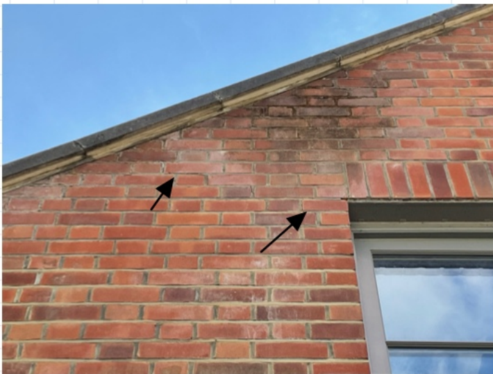
Cracking to front elevation at high level
