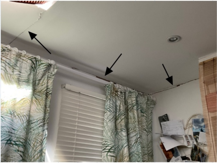
Cracking in ground floor front bedroom
