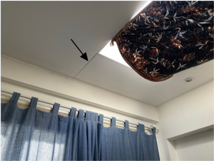
Cracking in ground floor front bedroom
