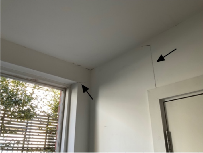
Cracking in hall
