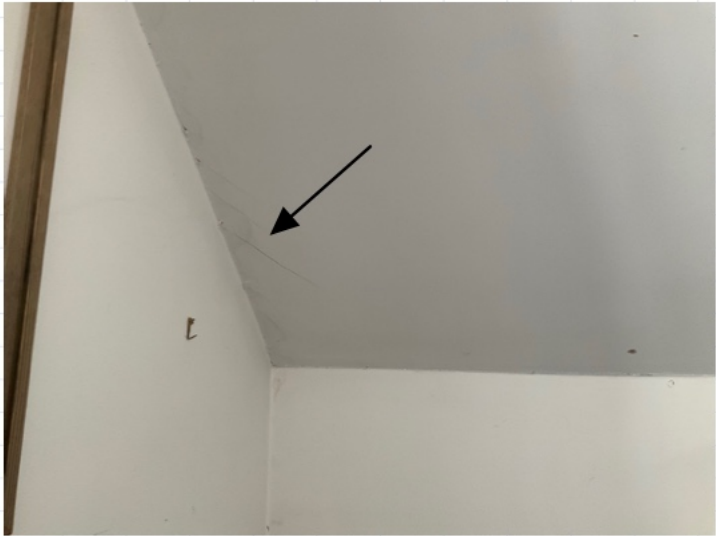
Cracking in 1st floor front bedroom
