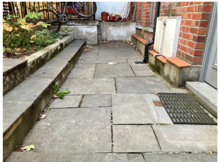
Uneven paving slabs along front of property
