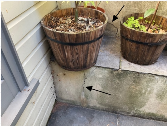
Cracking to boundary wall in courtyard area
