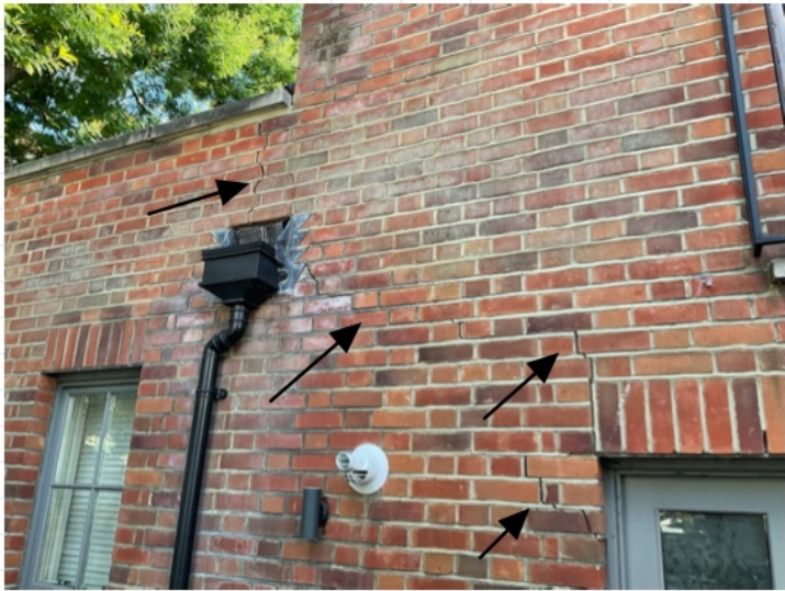
Cracking to front elevation
