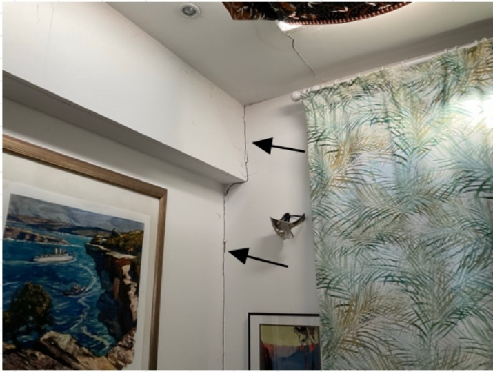
Cracking in ground floor front bedroom
