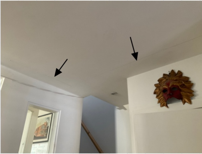
Cracking to ceiling in hall
