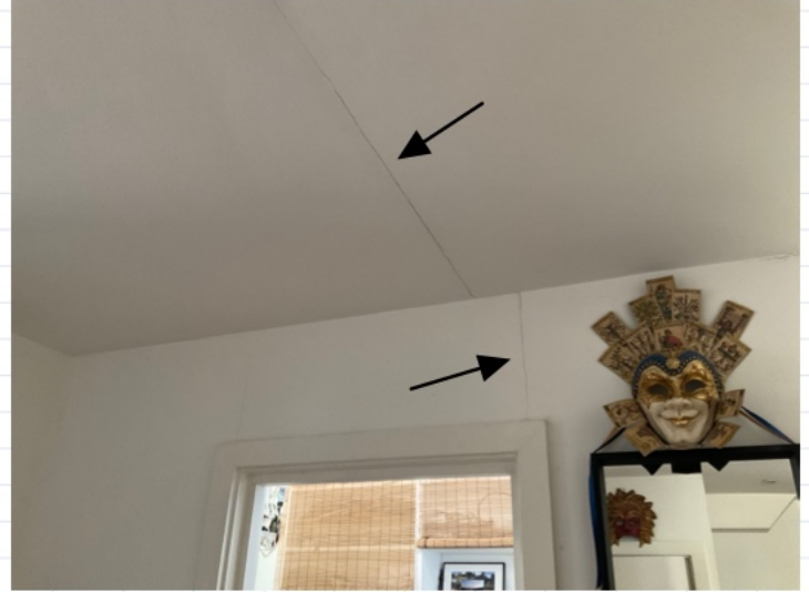
Cracking in hall
