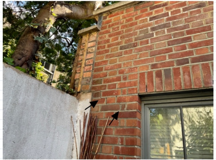
Cracking to front elevation
