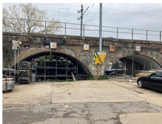
Photo 8: the series of rail arches provided no PRF.
