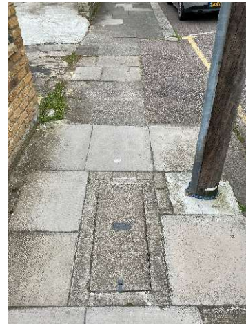
Photo 16 Footway cracking, utility cover surround damaged
