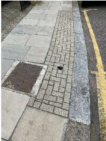
Photo 15 Utility cover surround damaged
