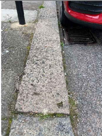
Photo 31 Sunken gully cover
