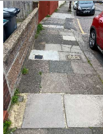
Photo 32 Footway cracking, footway scarring
