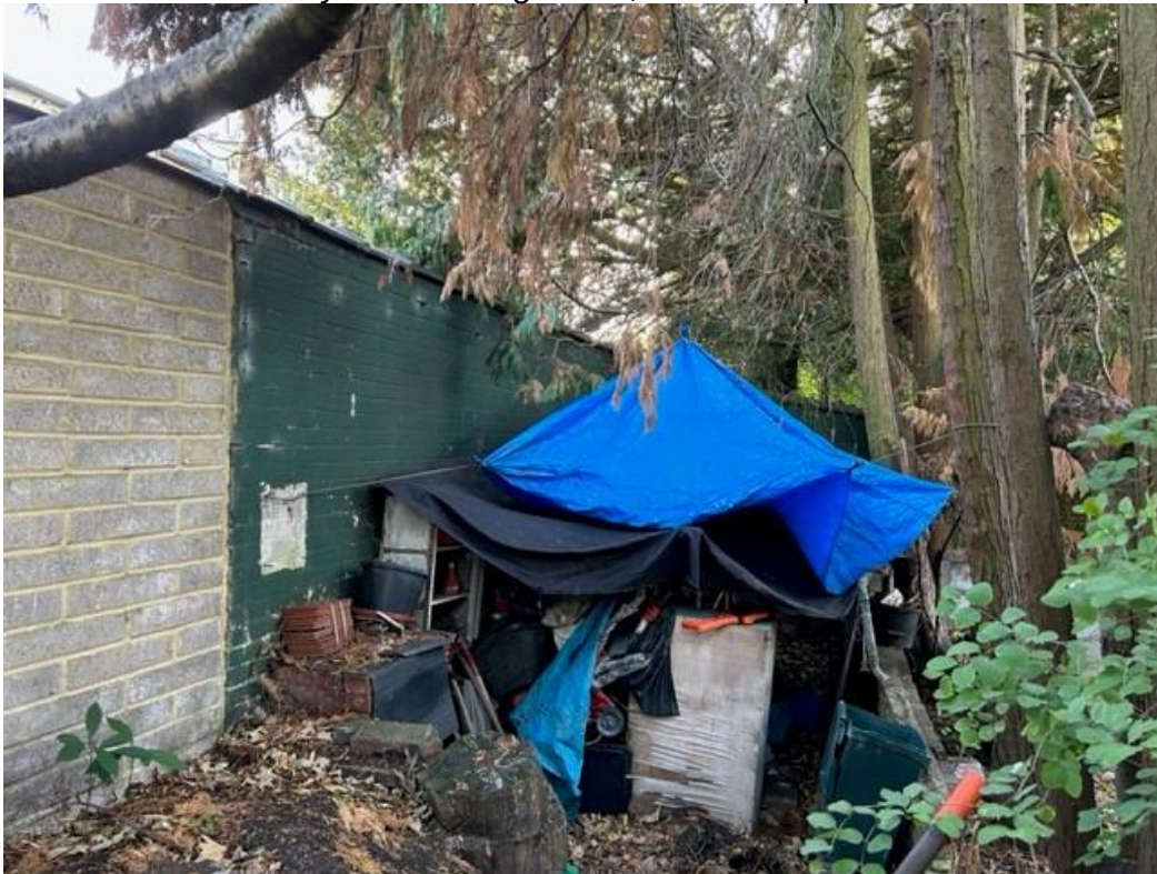
View of the boundary wall looking south, to the dilapidated shed.
