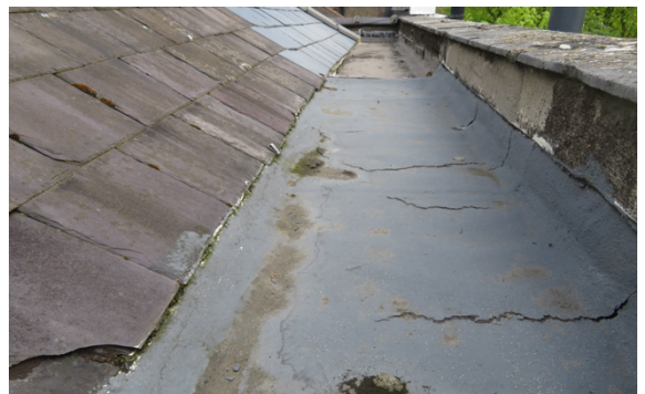
Failure of the recent overcoating of the asphalt to the front gutter
