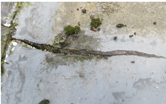
Deep cracks in the asphalt linings
