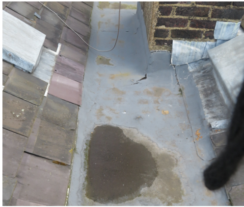
Centre valley looking north. Note the extensive disturbance to slating.
