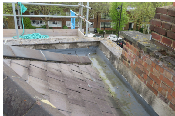
The hipped end of the front roof looking east. Note the Portland stone coping to the front parapet and disturbance to the slating.
