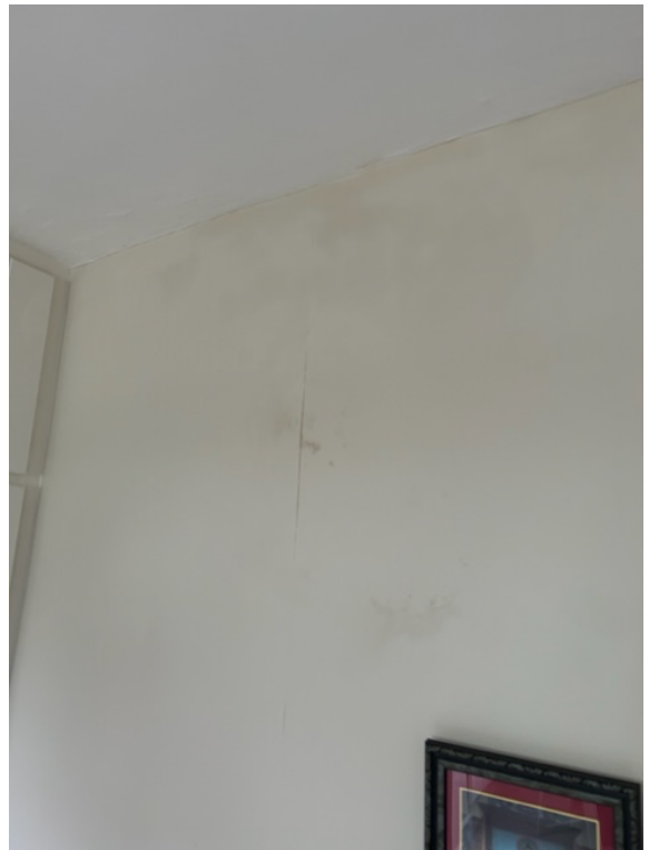
Damp staining extending onto second floor walls.
