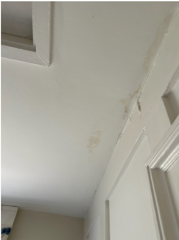
Damp staining on second floor ceilings.
