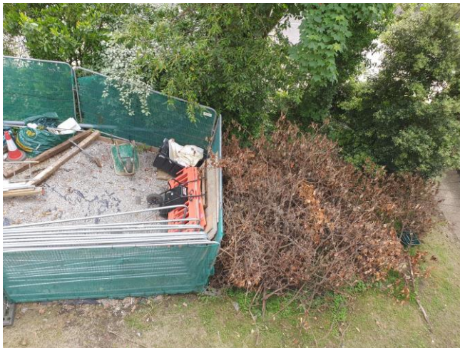
Photo facing towards Stanhope Road. Note the large amount of dead vegetation and plants that was cut/killed by the applicant during the construction of the penthouses. This became pest infested and after two years of being ignore by the applicant was cleared at the cost of the resident/flat owners. The dead vegetation took a whole day for waste contractors to clear. For scale the dead trees take up almost half the width of the entire front block.
