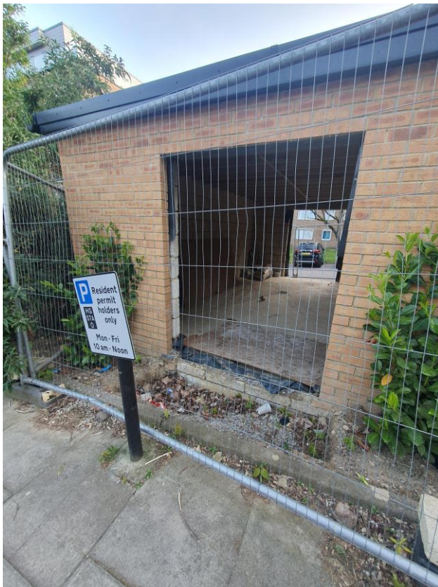
Close up of abandoned bike/bins shed view from the public pavement.
