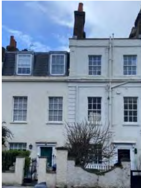
Figure 1 - Front chimney stack on left hand side has significant lean inwards
