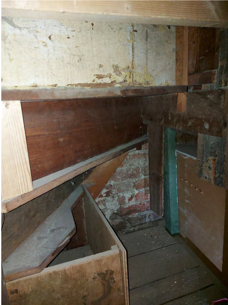
Fig.7: The upper winders of the upper stair, made of odd pieces of modern timber with some plywood.
