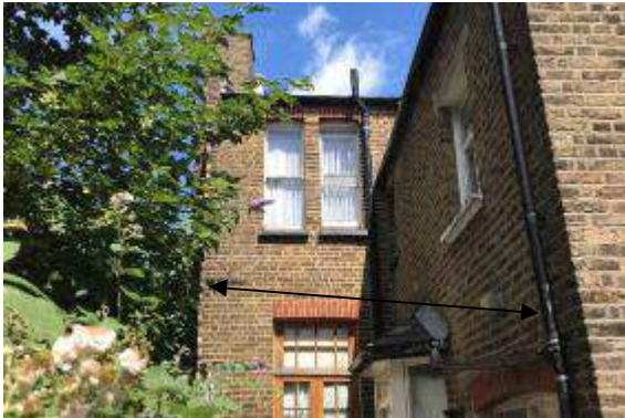
Neighbour (St Marys Church) Sycamore Tree 4m proximity from area of damage.
