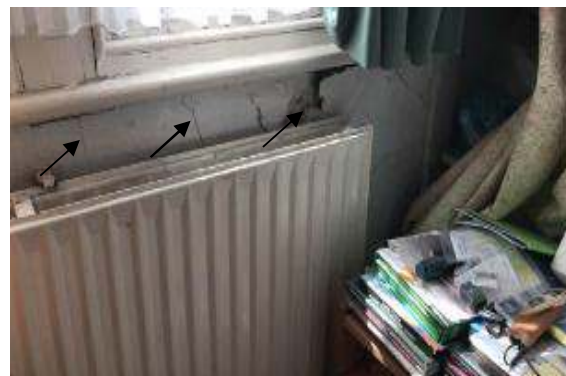
First Floor Rear Right Bedroom. Delamination of wallpaper, historic in nature and not indicative of subsidence.
