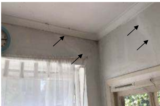
Rear Elevation Kitchen – Outrigger Ground Floor. Hairline cracks historically repaired. Not indicative of subsidence.
