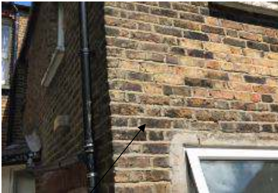
Rear Elevation Outrigger – Ground Floor. Stepped cracking through 8 courses of brickwork.
