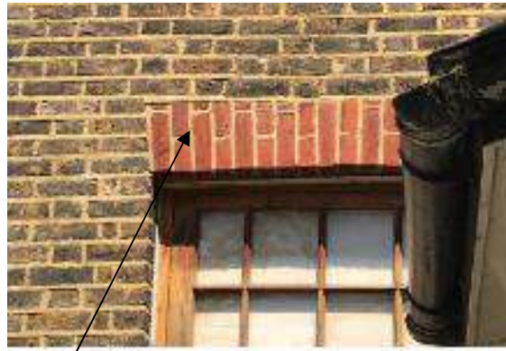
Rear Elevation Main House – Ground Floor. Hairline crack through soldier course and 2 brick courses above.
