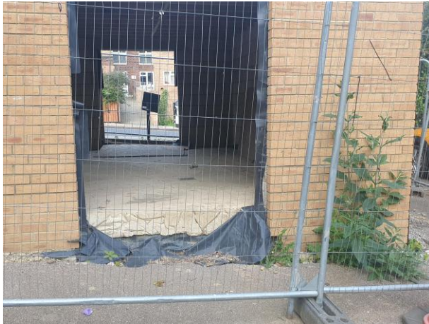
Close up of abandoned bike/bins shed view from the car park. Note the weed growth the site has been untouched for so long.
