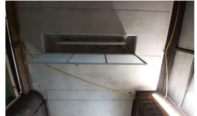
89B G.49 Vestibule ceiling radiator lights
