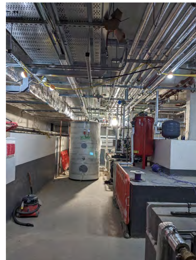
65A LG.43 Plant Room beneath Assembly Hall 2
