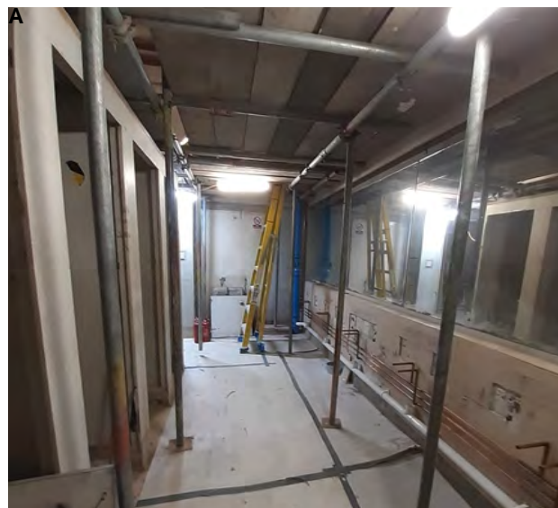
92 G.54 Ladies Lavatory looking back to entrance door
