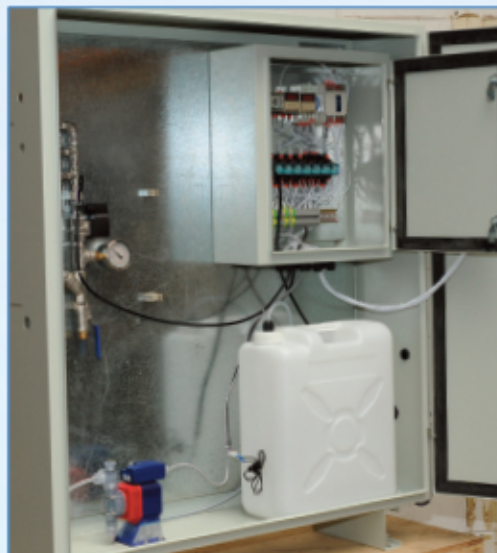
INTERIOR OF AUTOWASH CABINET
