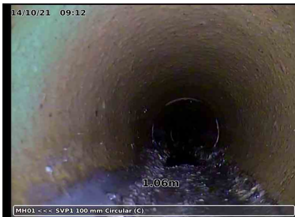
SVP1X_3279481a-6ebf-45f4-9add-3eb2347fad0f_20211022_125852_614.jpg, 00:00:31, 1.06 m Attached deposits, fouling from 4 o'clock to 8 o'clock, 10%
