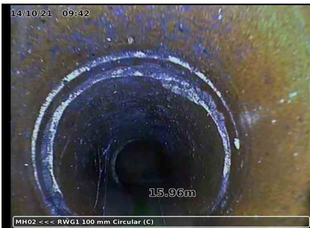
RWG1X_d583655e-defa-4b63-ba67-2d9d5e2d6ecb_20211022_131816_478.jpg, 00:04:18, 15.96 m Fracture, circumferential at joint from 8 o'clock to 3 o'clock
