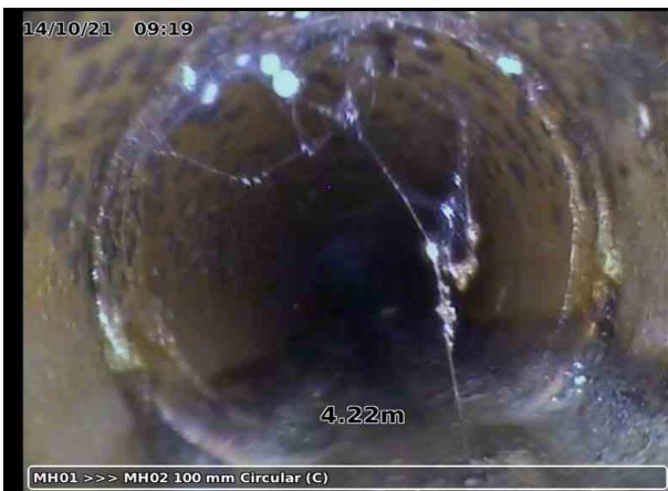
MH01X_fa3bcc3c-5db5-4e46-bf14-4a3987bf9fd1_20211022_130600_679.jpg, 00:01:13, 4.22 m Crack, circumferential from 2 o'clock to 9 o'clock
