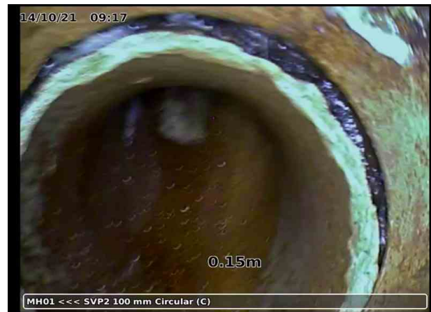
SVP2X_0a6b6b05-b783-422c-a79e-3e20b094f40f_20211022_130152_770.jpg, 00:00:07, 0.20 m Joint displaced, medium
