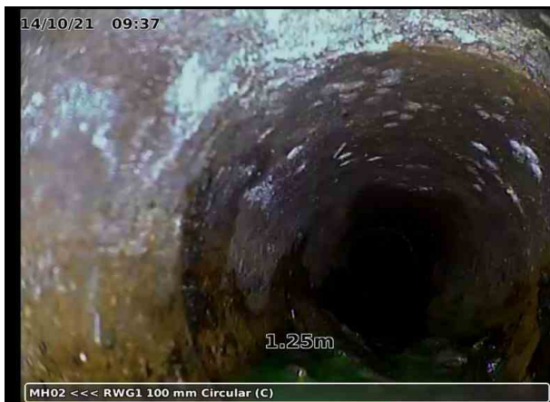
RWG1X_4afa57d1-a2a6-4006-9afd-5d33a941c063_20211022_131215_028.jpg, 00:00:21, 1.25 m Settled deposits, coarse, 10% cross-sectional area loss, start
