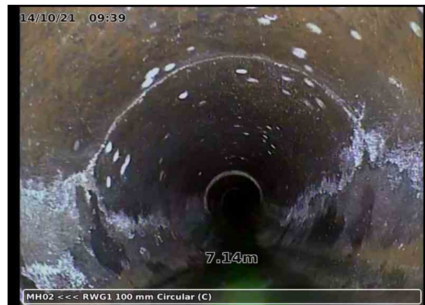
RWG1X_cc64321a-3fd3-4177-847a-eb47fd4d81d5_20211022_131454_008.jpg, 00:02:01, 7.14 m Crack, circumferential from 8 o'clock to 3 o'clock
