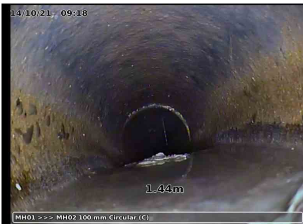
MH01X_95c10f1f-f9dc-46dc-ab4a-b366b9cac30f_20211022_130502_471.jpg, 00:00:32, 1.44 m Attached deposits, fouling from 4 o'clock to 8 o'clock, 20%
