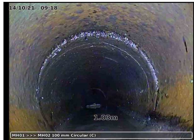
MH01X_40a3c49b-4962-4c0f-bb8d-987e9e914974_20211022_130436_754.jpg, 00:00:20, 1.03 m Crack, circumferential from 9 o'clock to 3 o'clock
