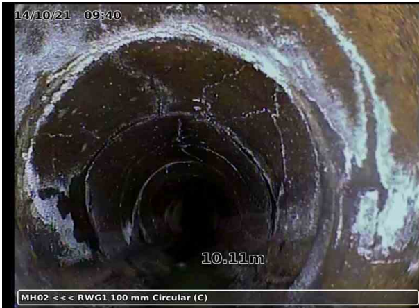
RWG1X_cabd6cdf-c75f-408e-8e86-cf633b5b3d51_20211022_131612_092.jpg, 00:02:50, 10.11 m Fracture, multiple from 12 o'clock to 12 o'clock, start
