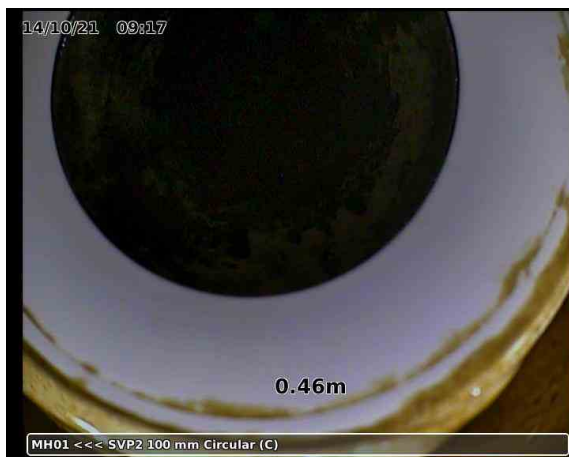
20211014-091654-snap0001.jpg, 00:00:17, 0.46 m Survey abandoned, REDUCER
