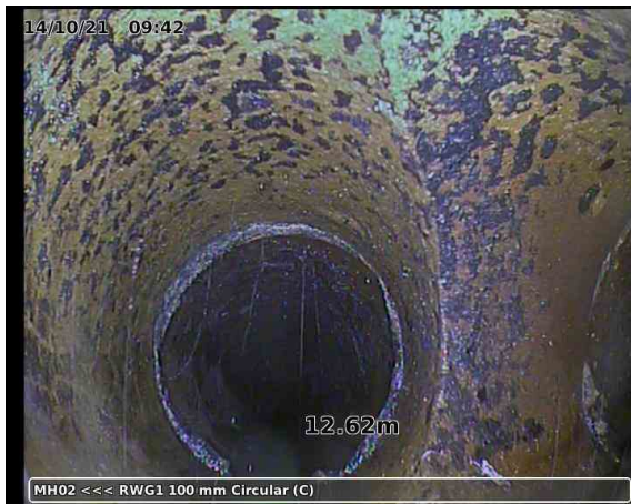
20211014-093650-snap0003.jpg, 00:03:37, 12.62 m Junction at 3 o'clock, diameter: 100mm, RWG3 RECESS RWG
