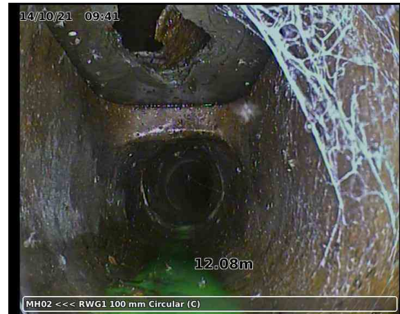
20211014-093650-snap0002.jpg, 00:03:19, 12.08 m General remark, ACCESS WITH MH01
