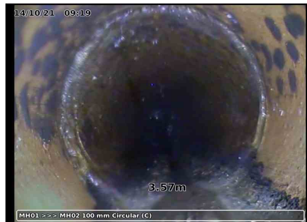
MH01X_127c206e-3bd1-4cde-be04-58b3ed858ab7_20211022_130538_274.jpg, 00:01:00, 3.57 m Joint displaced, medium
