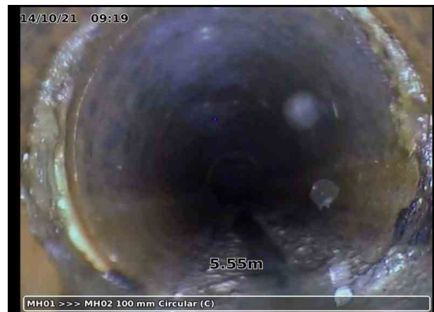
MH01X_3ab42e01-a17c-47f4-9851-177cd20dd02f_20211022_130637_479.jpg, 00:01:31, 5.55 m Joint displaced, medium
