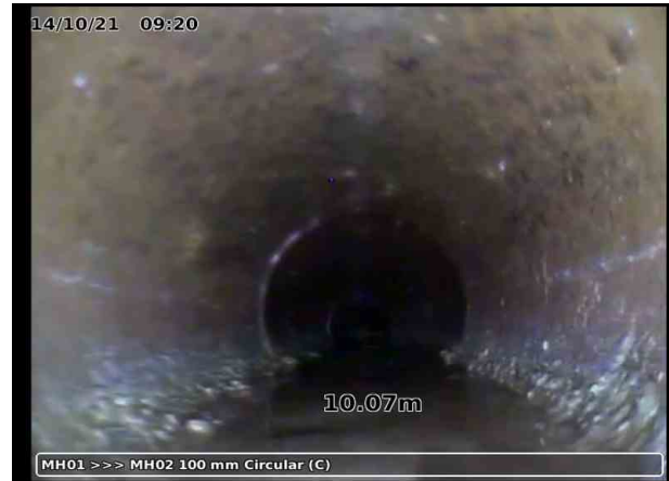
MH01X_22aa77ff-5750-454c-9cb3-709c4c8e094d_20211022_130923_143.jpg, 00:02:28, 10.07 m Attached deposits, fouling from 4 o'clock to 8 o'clock, 15%
