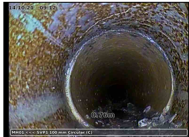
SVP1X_6ae17ec4-0410-47f2-bb4d-7cc238f35450_20211022_125822_076.jpg, 00:00:22, 0.76 m Cracks, multiple from 10 o'clock to 3 o'clock
