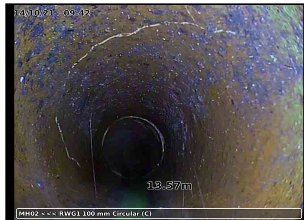
RWG1X_0cad6a68-50c9-4388-9716-e4322f79b848_20211022_131737_055.jpg, 00:03:48, 13.57 m Cracks, spiral from 7 o'clock to 1 o'clock
