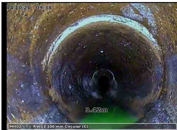
RWG1X_ad2f2bef-33b2-4de1-8ac0-2b11f80f40b4_20211022_131333_502.jpg, 00:01:08, 3.42 m Joint displaced, medium
