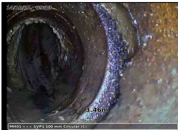
SVP1X_74e076ed-97d1-4dff-ad26-a122c59b6a12_20211022_125958_433.jpg, 00:01:10, 3.46 m Joint displaced, medium
