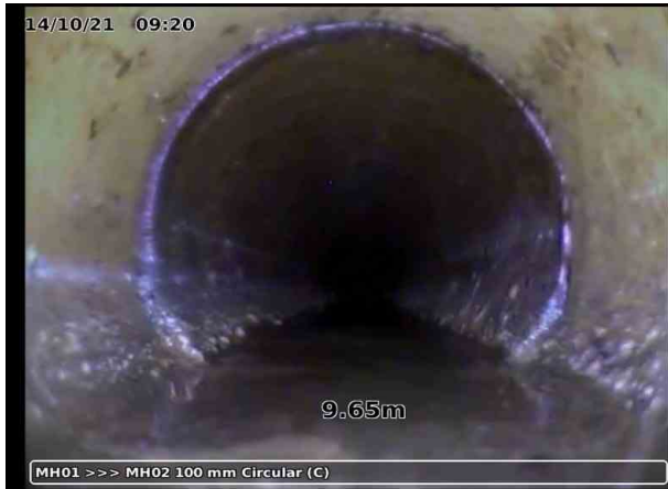
MH01X_eea5dcf7-03f2-49a5-8e33-85f122d42bae_20211022_130845_393.jpg, 00:02:23, 9.65 m Water level, 20% of the vertical dimension
