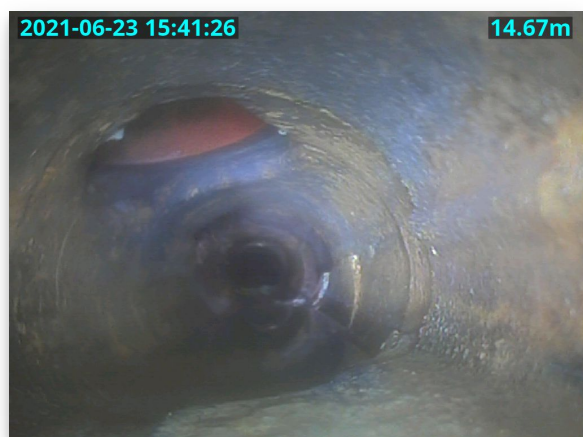
Fig 3.5: Line 4, cracking (Connection from clay pipe in MH2)
