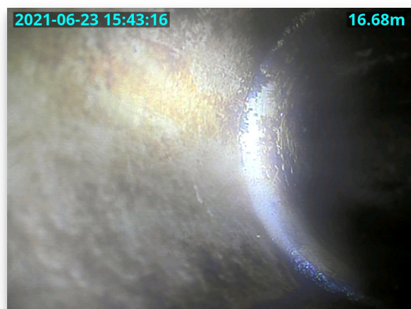
Fig 3.6: Line 4, joint displacement downstream from MH2
