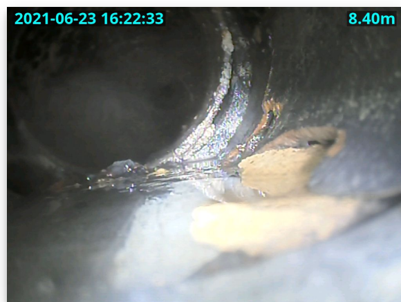
Fig 3.2: Line 6, hole in pipework
