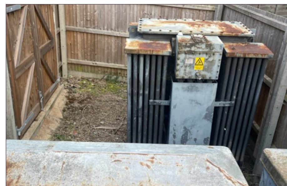
Neighbouring Sub-Station (over fence)
