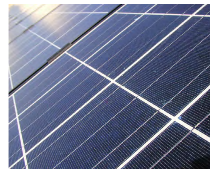
55. Photo Voltaic Panels
