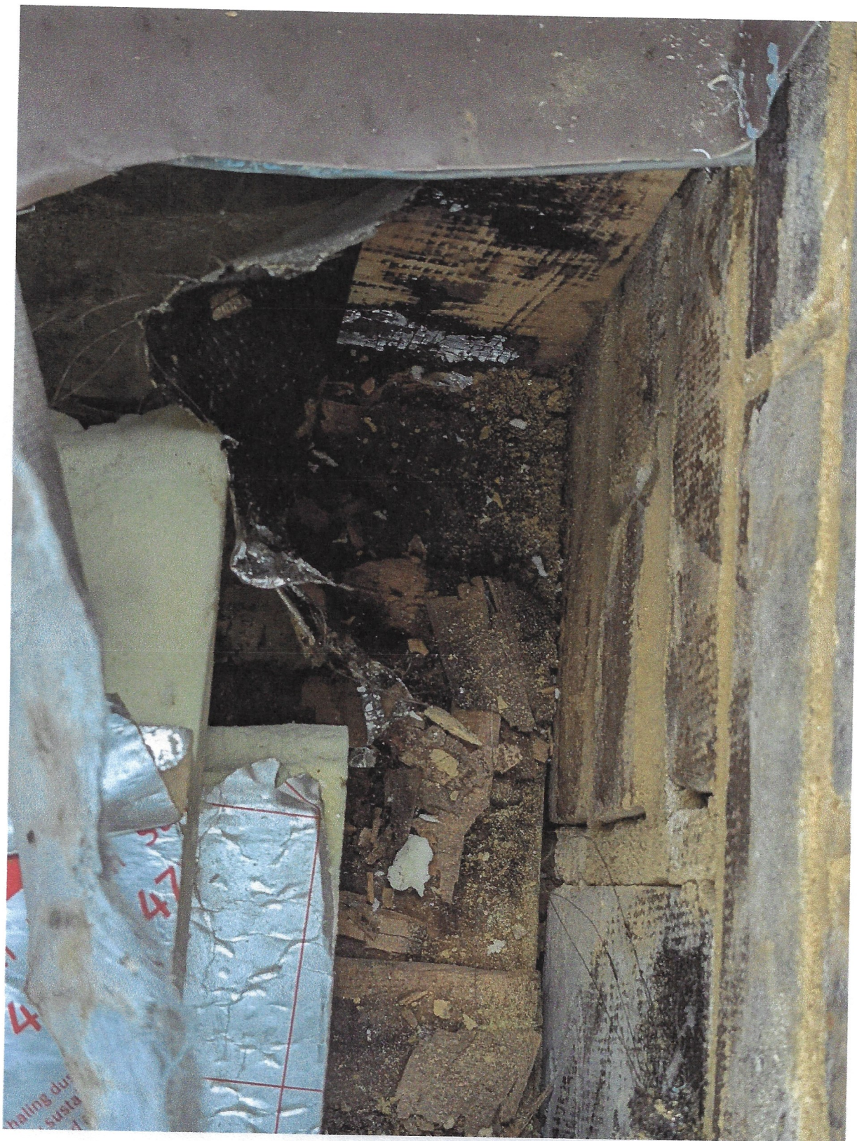
Water damage – southwest corner
