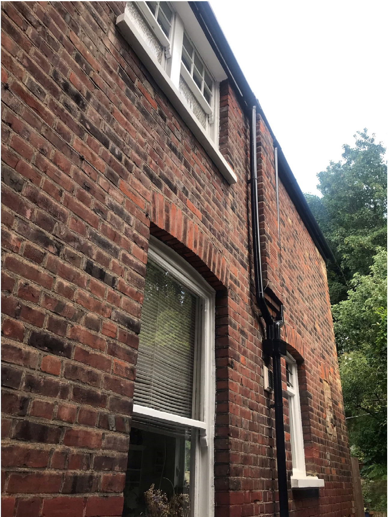
Image showing three of the 5 windows of No 32 that face onto the proposed flank wall (which will be just 1.59 metres away from No 30)
