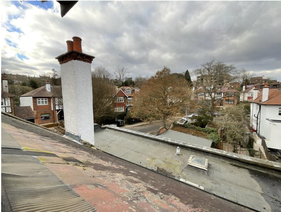
Poor condition of the existing roof
