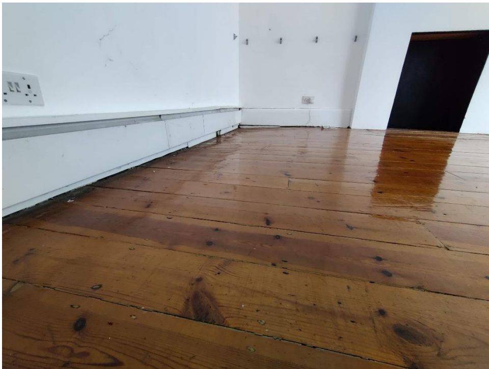
Uneven internal floors of 50 - 75mm differential across rooms
