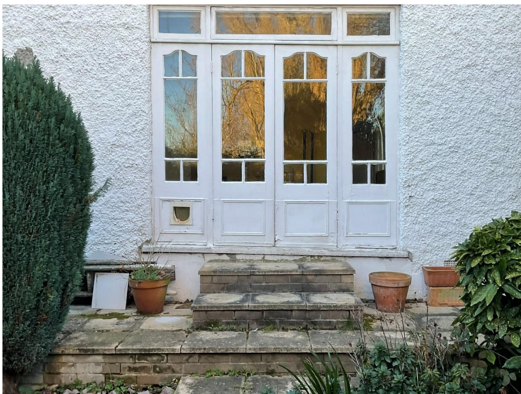
Evidence of structural subsidence, above right corner of patio door which is 70mm lower
