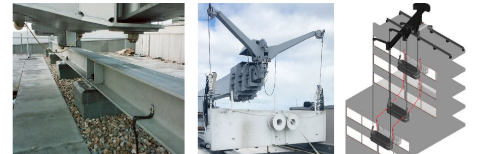
FIGURE 314. BMU external track and restraining soft rope spools
