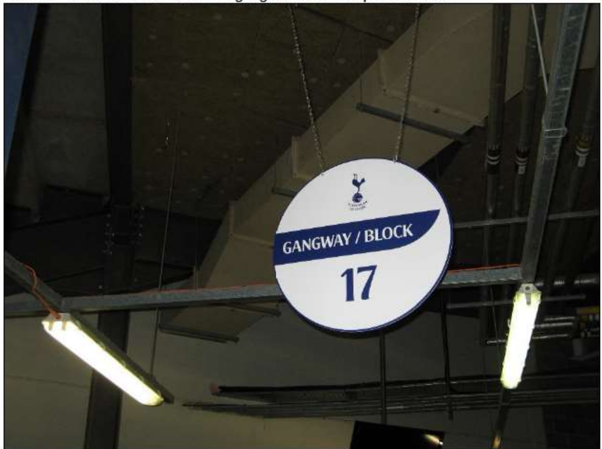
Photo H – location of this flue with signage in front to help find location
