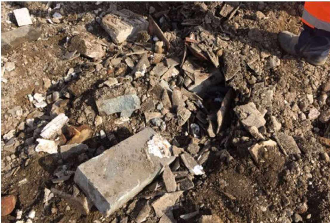
Figure 4-5 – Broken asbestos sheeting
