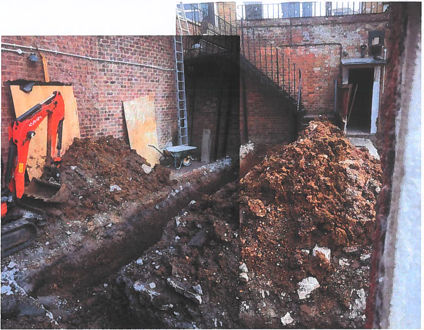
Above: Composite of Noisy digger and Blocked staircase entrance to No 78A
