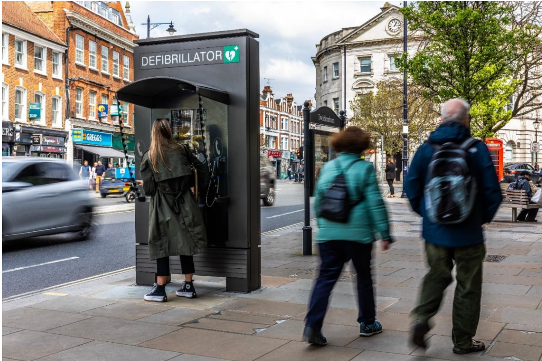
INSTALLED HUB UNIT IN TWICKENHAM
