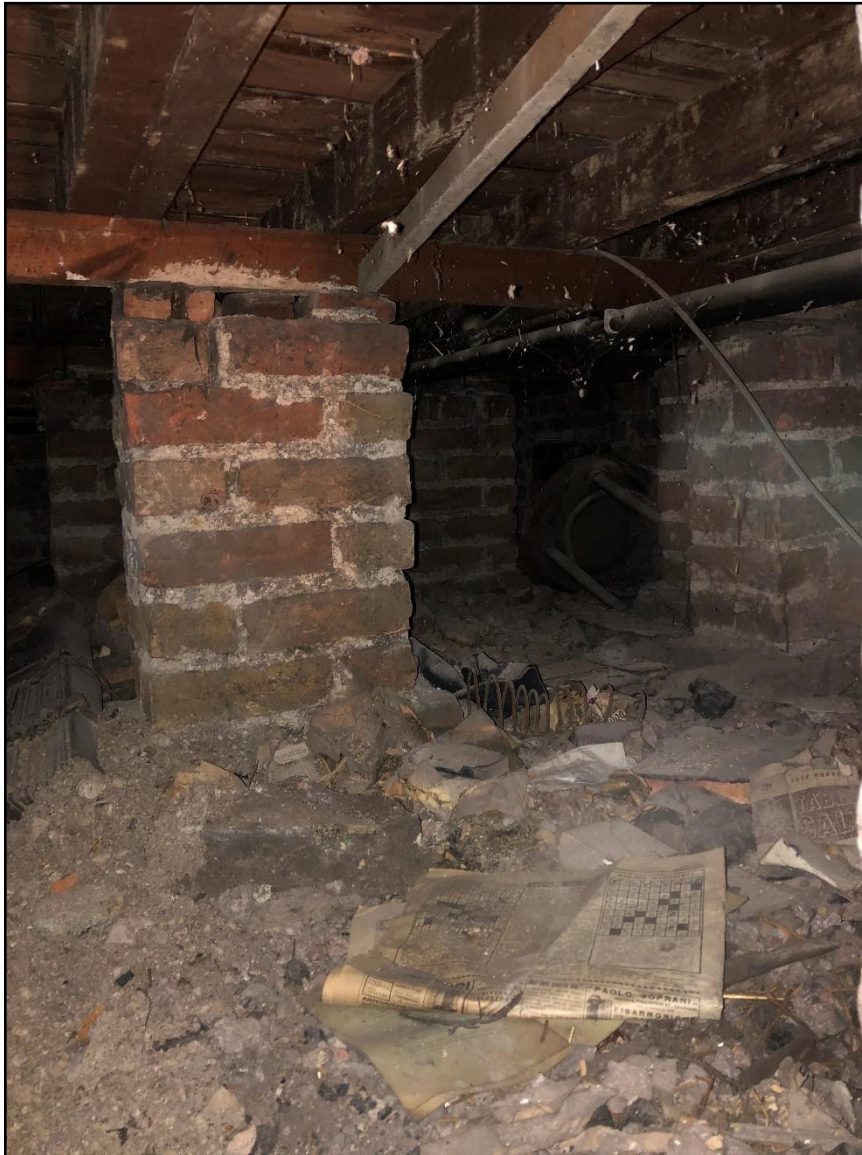
Photograph 4 – Void below floor where there is no cellar
