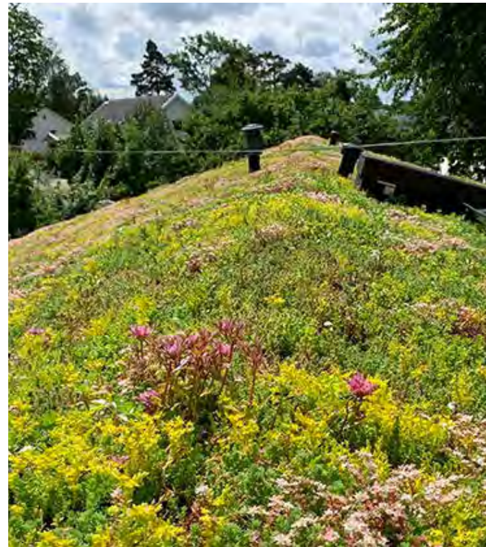
Sedum extensive green roof
