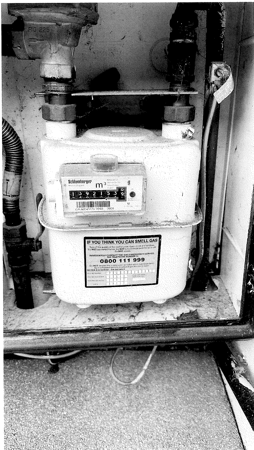
Gas meter for the Flat
