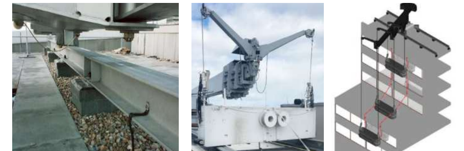
FIGURE 314. BMU external track and restraining soft rope spools
