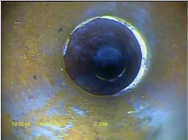
00:00:58, 7.20 m Medium displaced joint
