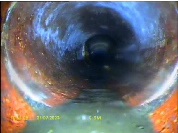
00:00:15, 0.30 m Medium displaced joint
