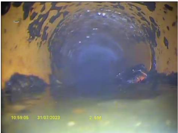
00:00:45, 2.50 m Medium displaced joint
