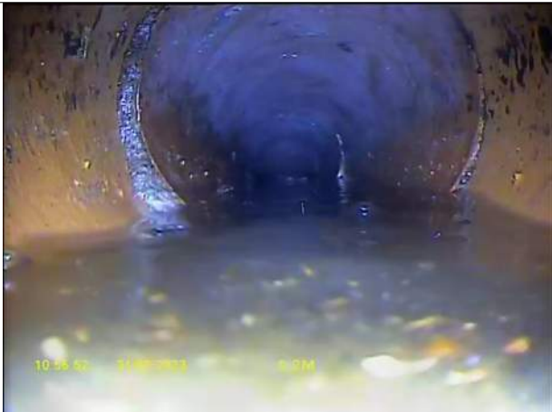
00:00:39, 5.00 m Medium displaced joint
