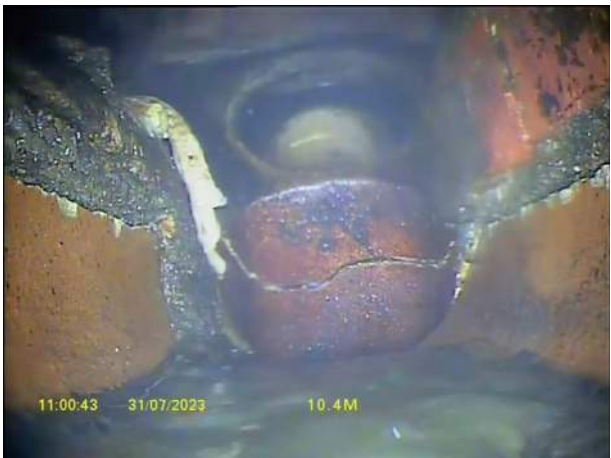
00:02:05, 10.50 m Finish winser trap, MH04, the pipe is failing to discharge
