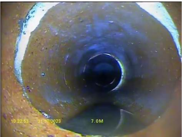
00:00:53, 7.00 m Water level, 5% of the height, Water pooling behind displacement. Can leak.
