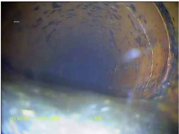
00:02:47, 2.40 m Circumferential crack from 1 o'clock to 5 o'clock
