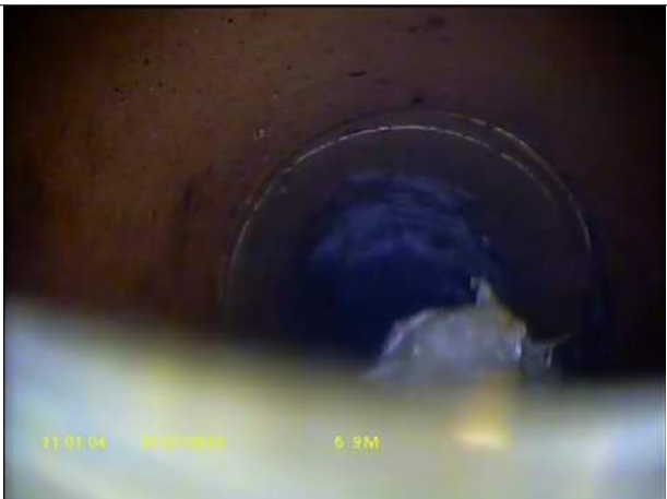
00:02:26, 7.00 m Circumferential crack from 8 o'clock to 4 o'clock
