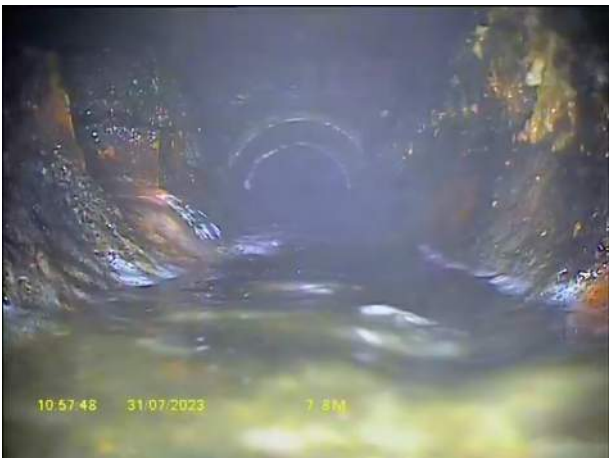
00:01:17, 7.50 m Finish manhole, MH03, the pipe is failing to discharge, Responsibility of LWA/Build-over agreement required. Public asset.
