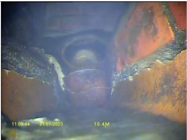
00:02:05, 10.40 m General remark, Winser Trap missing lid suggesting a history of blockages.
