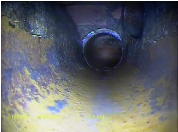
00:01:34, 15.60 m Finish manhole, MH00, the pipe is flowing fine, Responsibility of LWA/Build-over agreement required. Public asset.
