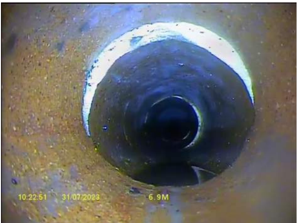
00:00:51, 6.90 m Medium displaced joint
