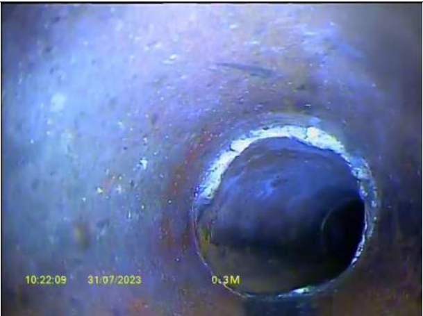
00:00:09, 0.30 m Line deviates right, quarter, 15 Degree bend
