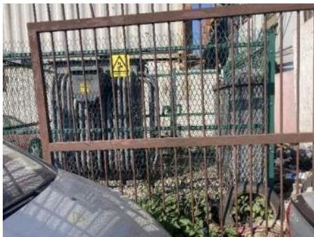
Figure 2-8 - Electricity substation located about 10m northwest of the Site.
