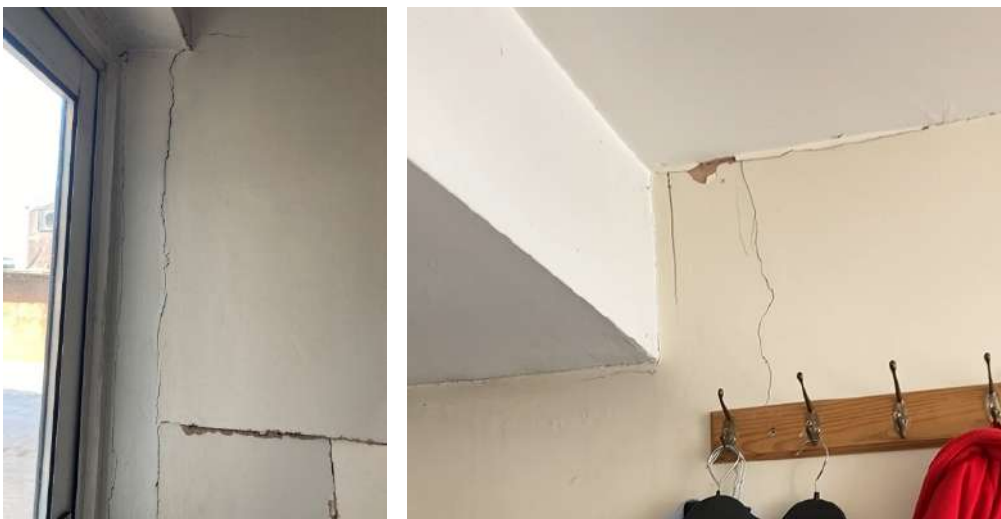
Figure 4-2 -Superficial cracking in finishes in Unit 812 b) Landing and c) Flat C
