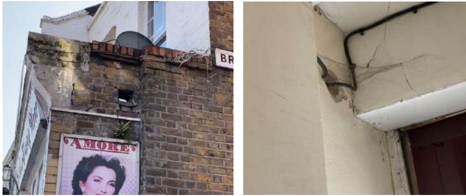
Figure 4-3 – a) localised cracking of brickwork to parapet of Unit 829, b) damage around drilling for conduits in hallway of Unit 821
