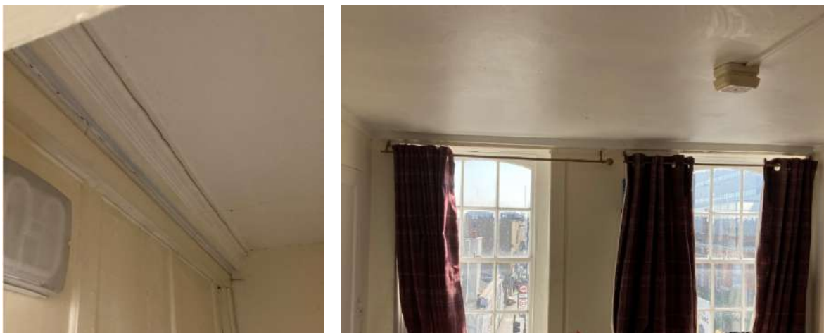
Figure 4-1 – a) Hall of Unit 823 with superficial cracking in finishes, b) perceived deflections over window line in Unit 819 Flat 3
