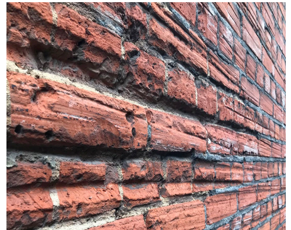
FIGURE 160. Damage to the Brunswick Square Brickwork
