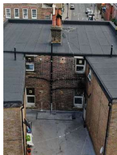
Figures 54 and 55 (above) – Typical cracked paint and poorly added services on the front elevation.
