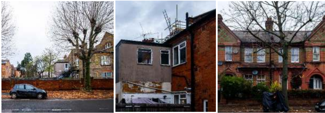
Figure 41. Several examples of the status of windows which need to be repaired. Source: SLHA@Dec'21.
