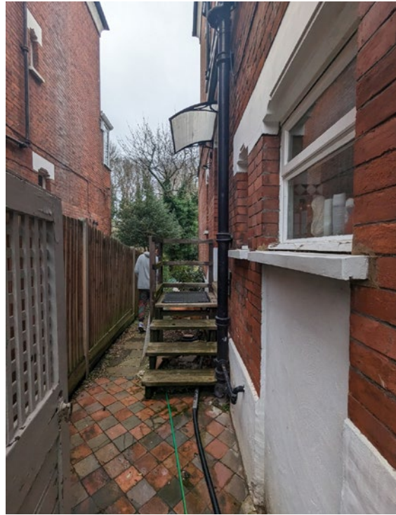
The existing rotting access stair to the current lower ground floor entrance and historic entrance floor tiling. The proposal is to remove the stair and relocate the entrance. A continuous new lower level would receive similar historical patterned tiling.
