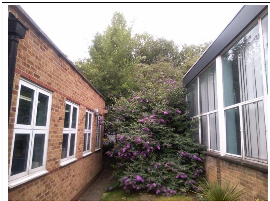
View of TG11 – lapsed shrub/scrub understorey in contact with building
