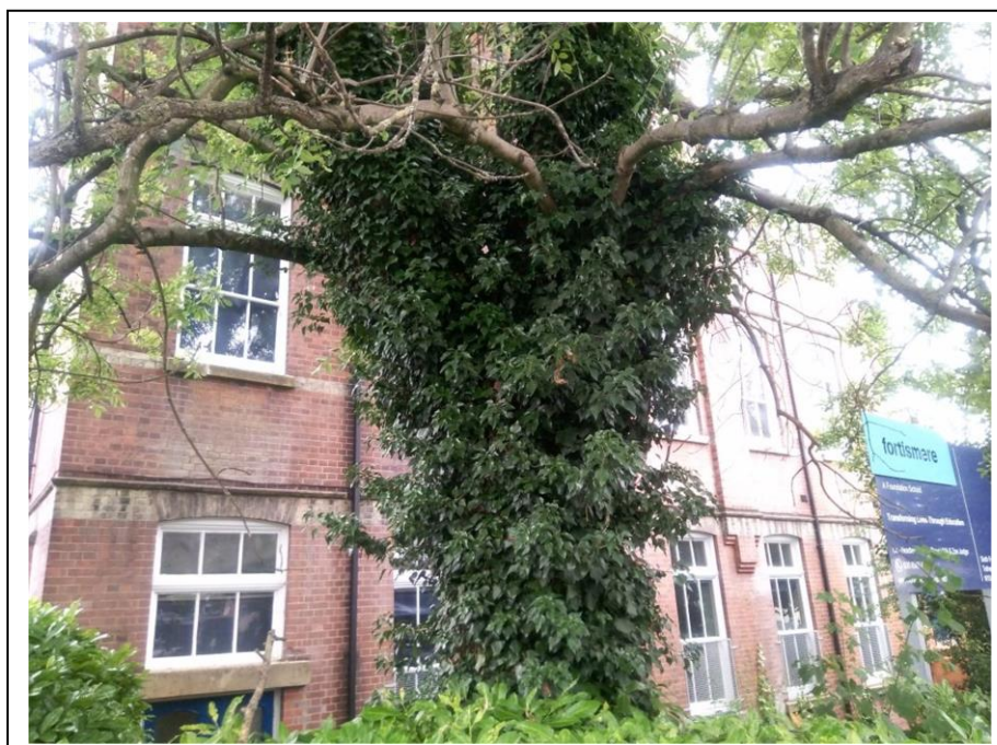
View of T51 Ash - extensive Ivy growth to main stem obstructs view of stem condition
