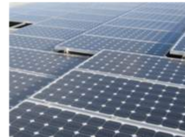
Solar PV system
