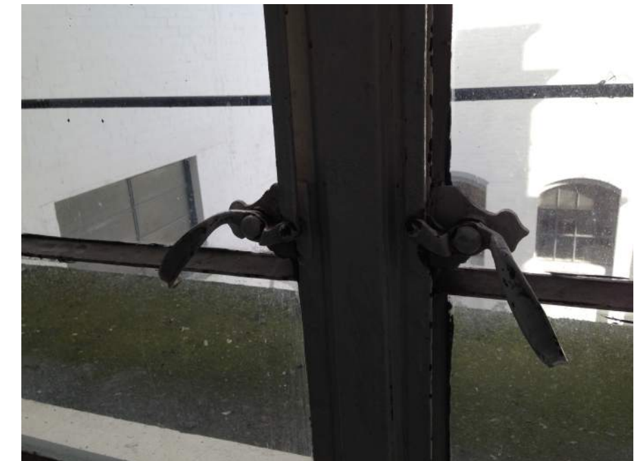
Many of the windows no longer seal internally letting cold air into the building and creating drafts.
