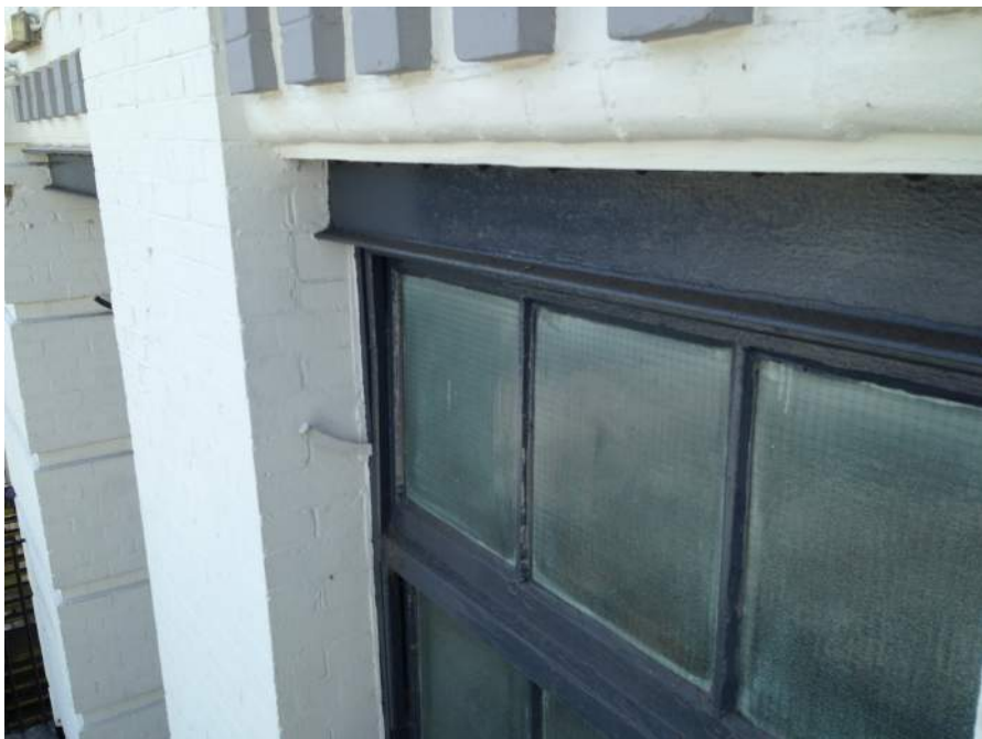
The steel lintel above windows is a major thermal bridge that will need to be addressed in the renovation works.
