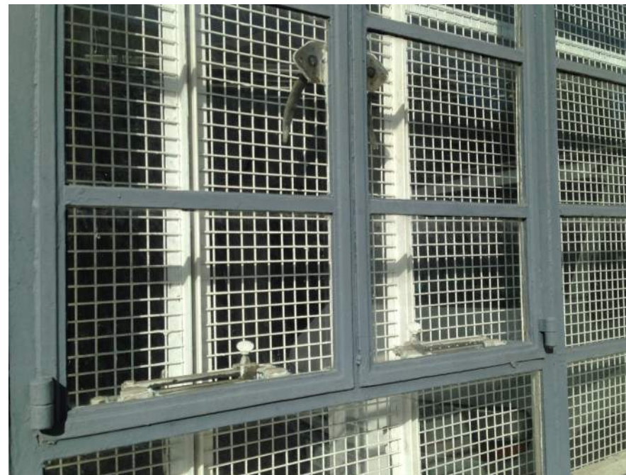
The steel windows have exceeded their working life and require replacement. The steel frame and single glazing has a significant impact on the internal environment.
