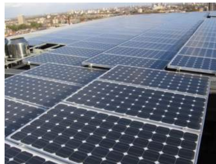
Example solar photo voltaic array
