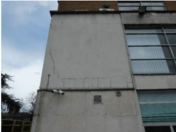
Photo 29: Render on North-West corner, with extensive cracking
