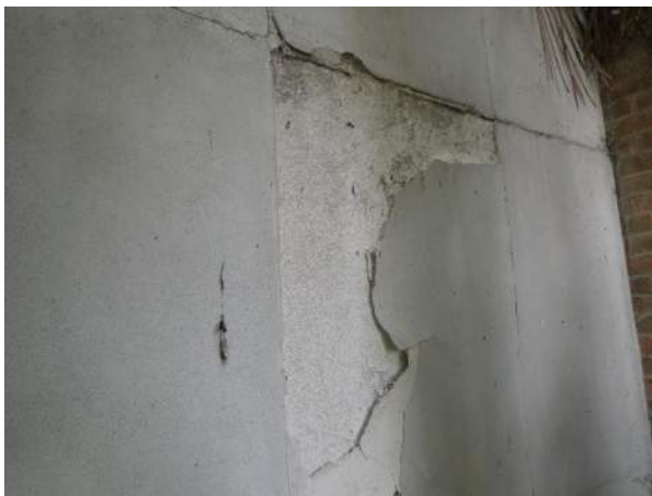
Photo 19: Patchy/peeling render on precast concrete panels adjacent to entrance
