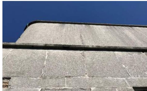
Photo 56: Crack in render on roof outbuilding
