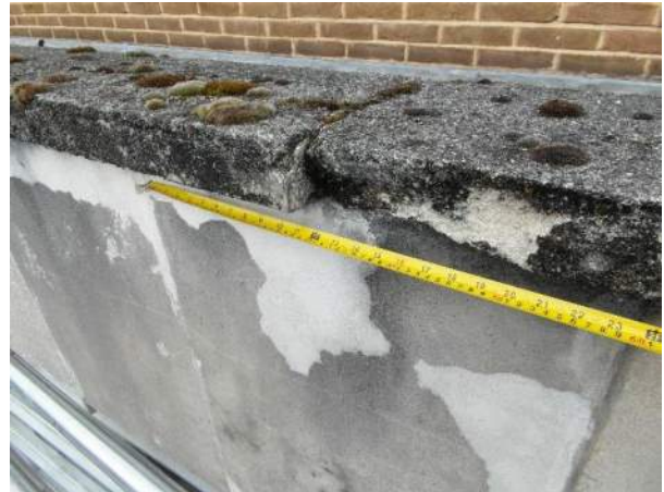
Photo 50: Degradation of stone coping above precast concrete cladding (with peeling render layer)
