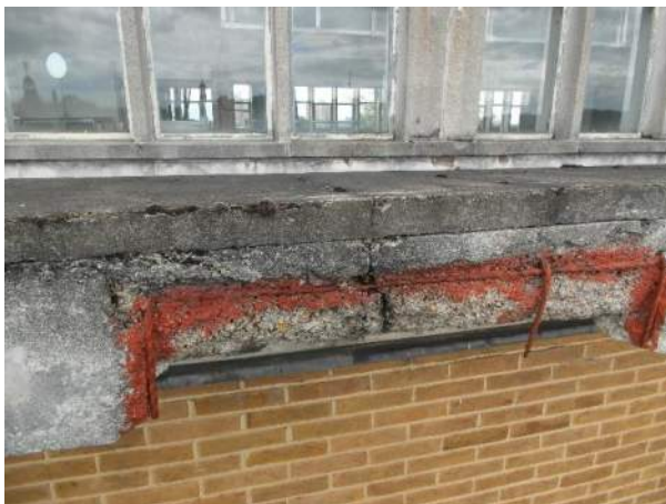
Photo 51: Example of failed cornice panels, with exposed corroded rebar (with red oxide paint previously applied)
