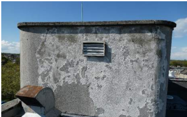
Photo 55: Render layer peeling off concrete wall
