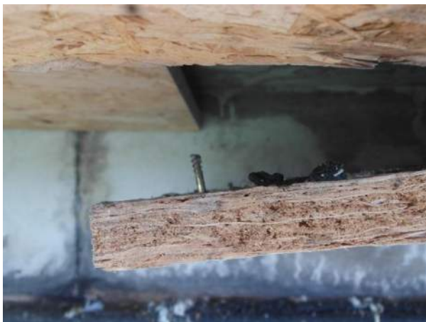
Photo 47: Example of failed fixing in Sterling boards installed
