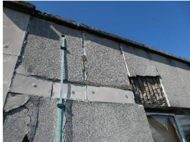
Photo 22: Extensive damage to precast panels at Level 3 (South elevation) with spalling/cracking and exposed corroded reinforcement
