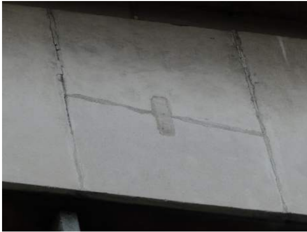
Photo 17: Cracking in precast concrete panels above curtain walling (main entrance) on East elevation
