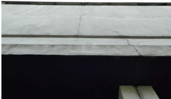
Photo 31: Cracking on North elevation of 'West Wing', at movement joint location
