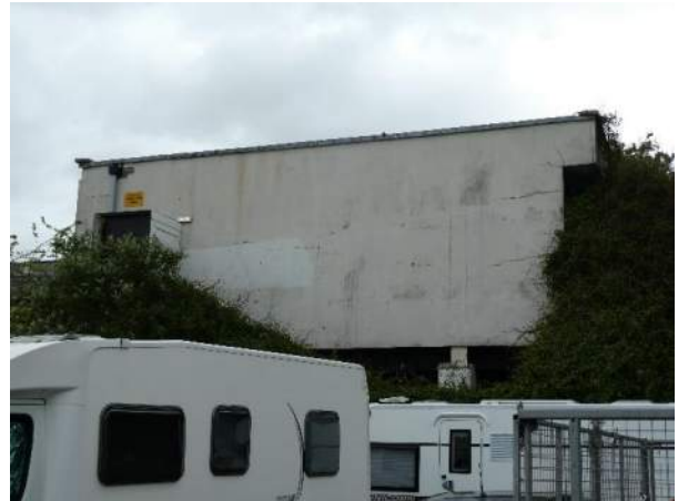
Photo 30: Render on West elevation of 'West wing', with extensive cracking, locations of primary structure highlighted through cracking
