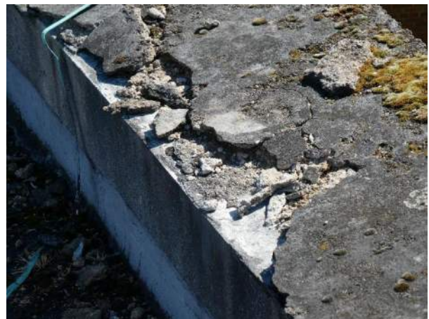
Photo 52: Degradation of stone coping on sky face
