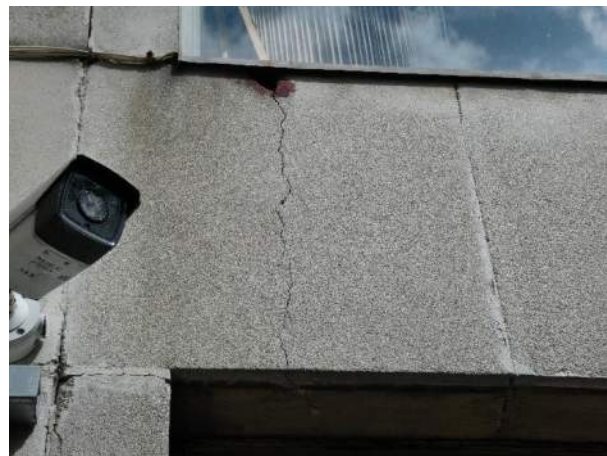
Photo 20: Cracking and exposed reinforcement (with red oxide paint) in precast concrete panels
