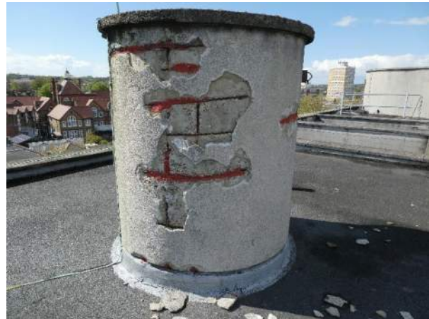
Photo 54: Boiler flue with extremely decayed concrete
