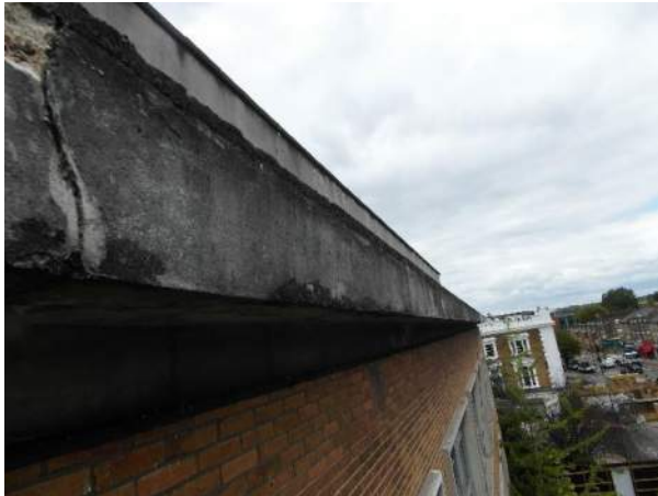
Photo 49: Degradation of concrete cornice above brickwork
