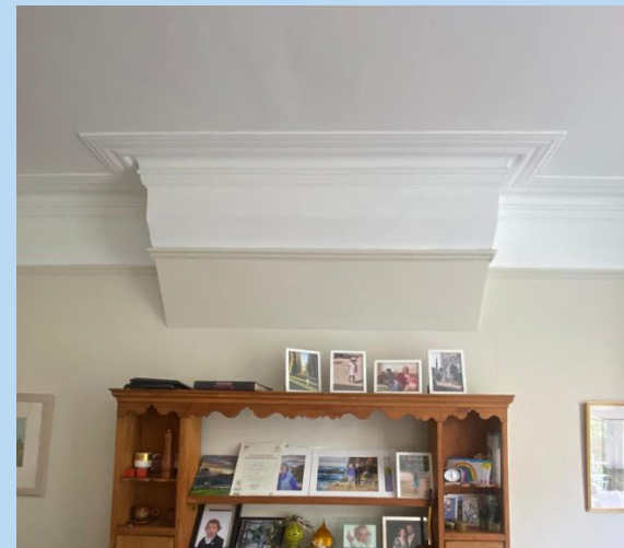
13 Lynmouth Rd - Ground Floor, a small portion of the chimney breast remains.
