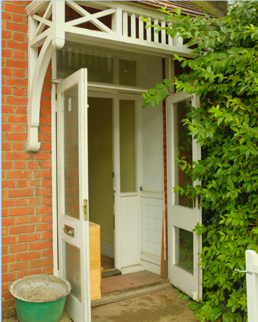
11 Lynmouth Rd (Application Property) - Entrance door pushed backwards.
