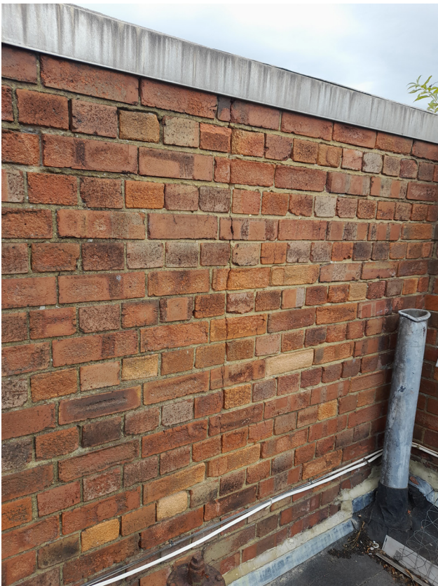
Crack to north parapet to be investigated as part of works.
