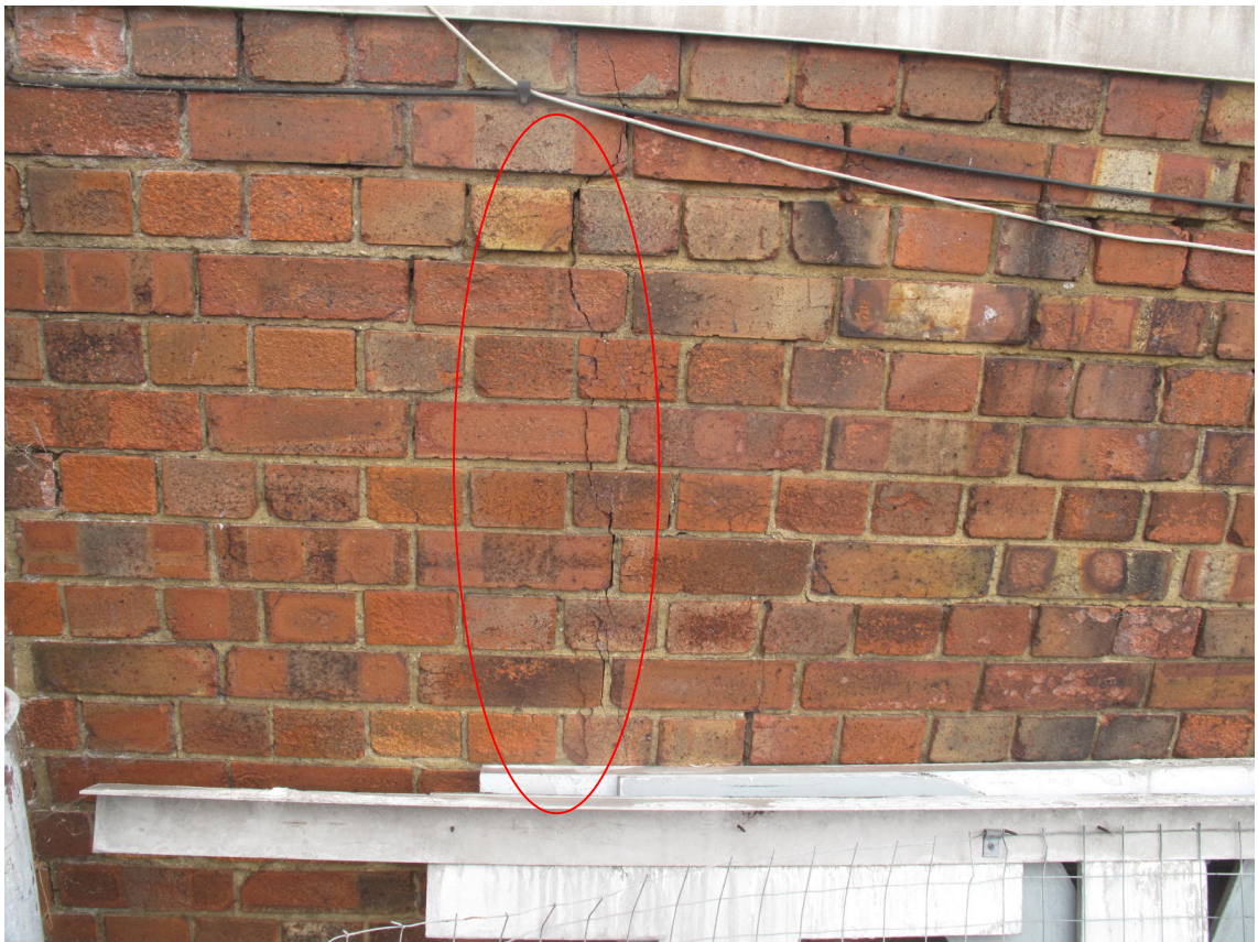
5. Detail of cracked brickwork to rear of front elevation to be investigated
