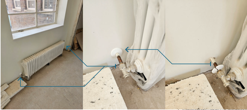
The radiators are consistent in finish and design across the building. An installed radiator in modern refurbished area is shown left. Pipework is hidden in the walls in all locations, with a single penetration at top and bottom tight to pipe with a cover cap to match finish of wall.
