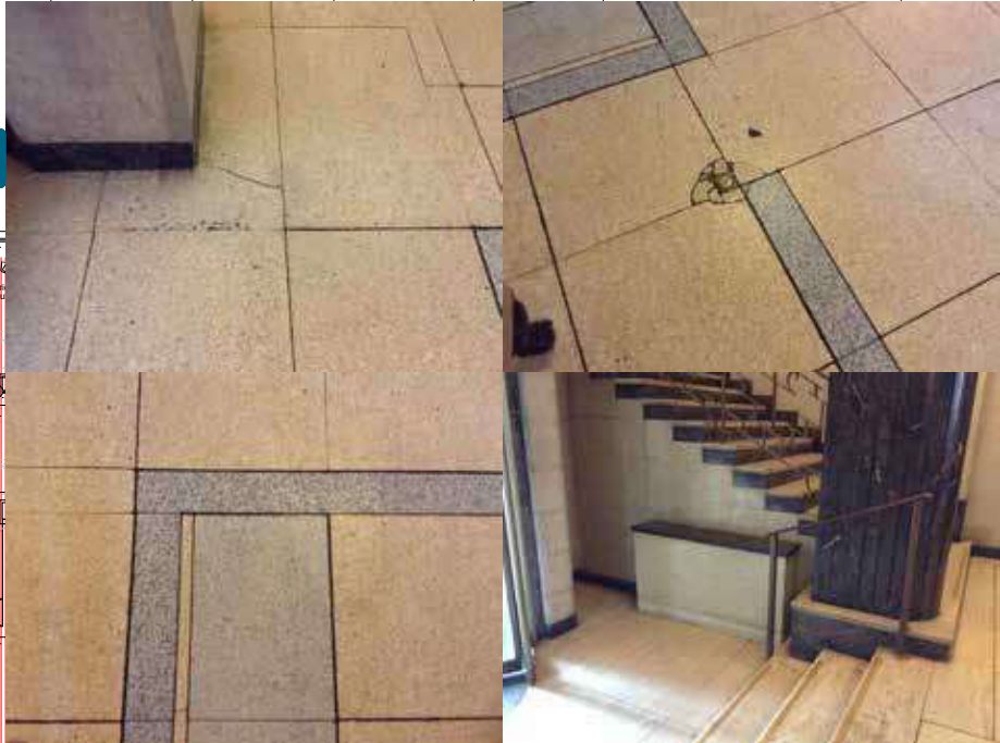
Entrance Foyers Both the entrance foyer and hall have terrazzo flooring with the foyer using a mixture of pale blue and cream tiles. Localised areas contain mostly hairline cracks with some tiles showing larger sections of damage. (The cracks are to be repaired and any tile beyond repair is to be replaced with a like-for-like finish as method statement ALT-411 and ALT-412
