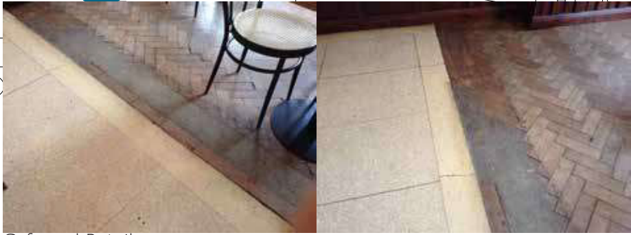
Cafe and Retail The lobby terrazzo floors run into the cafe and new retail area (formerly the Ladies Cloakroom), which is bordered with original herringbone flooring, within the new retail space, similarly to the lobbies the terrazzo shows mostly light damage with hairline cracks, light repairs are required as method statement ALT-411 and ALT-412. The existing timber is also heavily worn and scratched, this is to be refurbished as method statement ALT-538.
