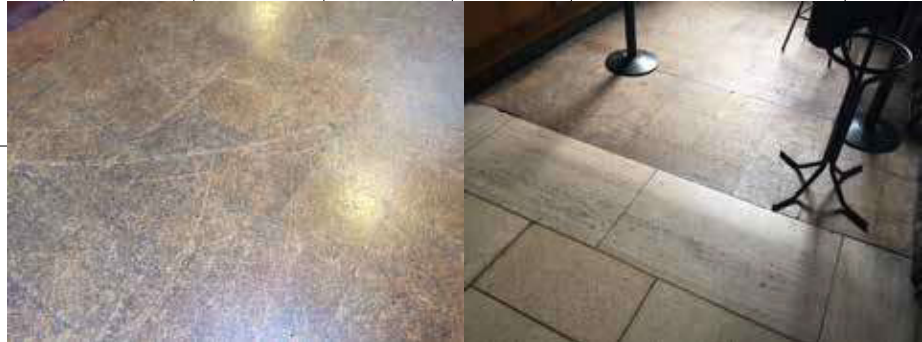
Hallway and Co-working Space Original cork flooring previously hidden under more modern coverings with the cork showing signs of degradation and wear. The modern coverings have been removed and the cork floor is to be repaired as ALT-511
