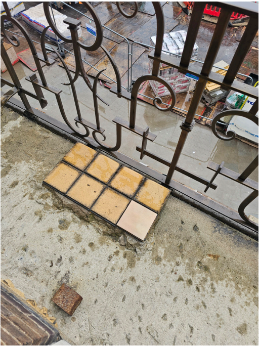
Existing tiles on balcony are to be replaced with new like-for-like replacement tiles.
