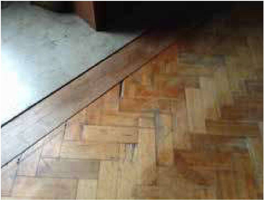
ALT-415 Stone Floor Repairs Stone borders to perimeter of flooring. The stone is generally in good condition but appears worn with some hairline cracks - to be refurbished as relevant method statement.
