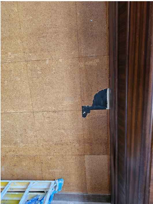
ALT-559 Refurbishment of veneered wall lining Existing cork wall shows signs of wear, a sample of refurbishment has been approved on site (as bottom right panel). The cork is to be repaired in situ and where significant damage to tiles as middle right hand side, tiles are to be replaced with matching tiles as the approved sample
