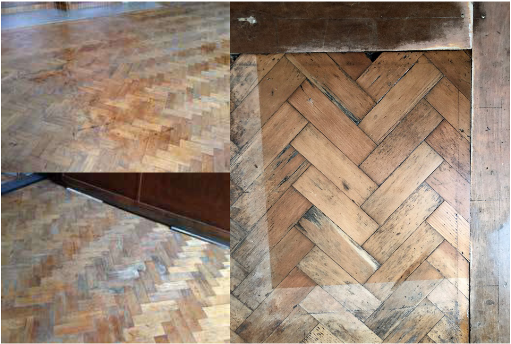
ALT-535 Repairs to Herringbone Flooring Existing timber herringbone flooring had localised damage that was apparent with areas heavily scratched and surface inconsistencies with marks and stain - the refurbishment of the flooring is bring the floor up to a good quality while maintaining its aged appearance.
