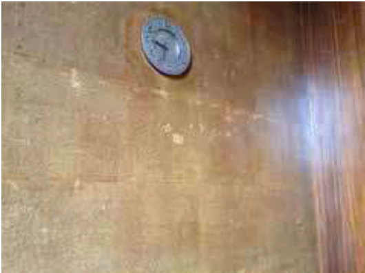
Original clocks are at opposite ends within the cork walling. The clocks were previously wired and connected to the Synchronome master clock. Due to the relocation of the clock to a central location on the
