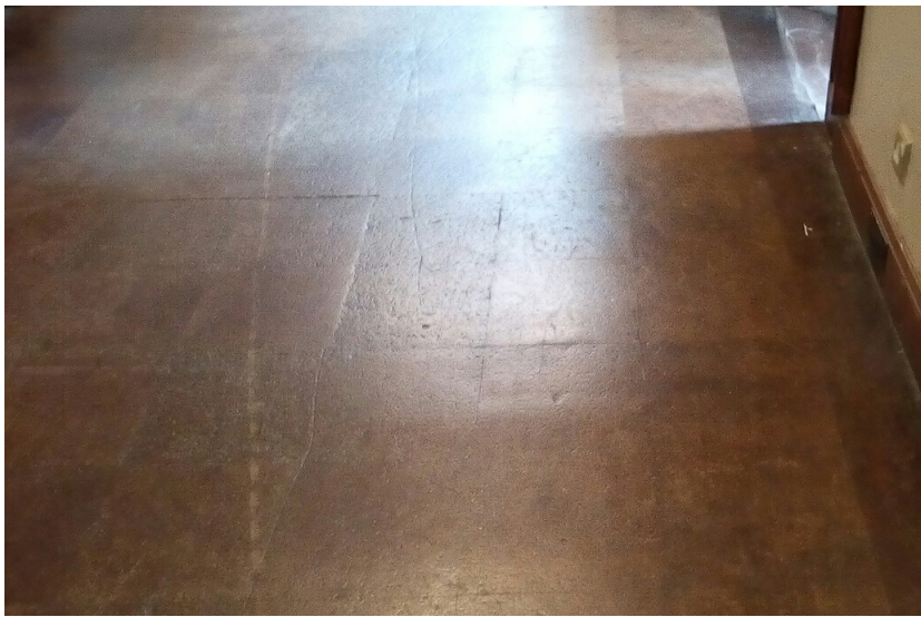
Original flooring displays wear and tear with some scratched, cracks and dents throughout, it is to be repaired to the approved samples as relevant method statement ALT-515
