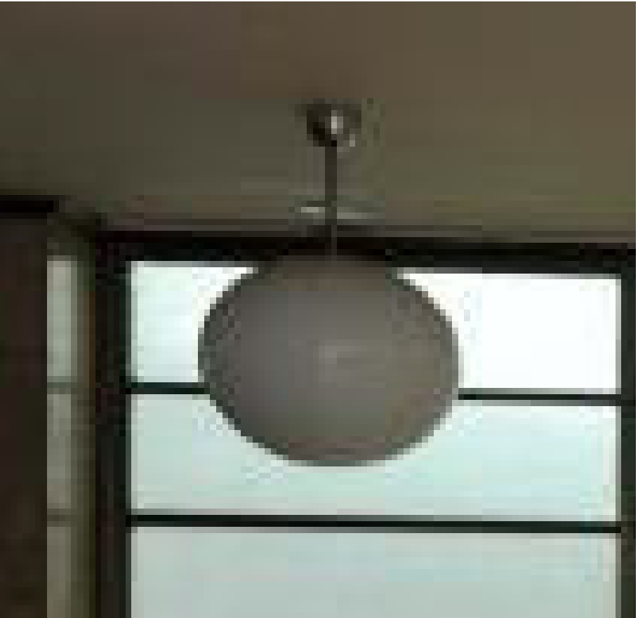
Existing globe pendent are to be refurbished, relamped and reinstated in existing positions.
