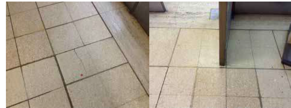
ALT-411/412 - Terrazzo Floor and Skirting Repairs Existing terrazzo flooring is made up of cream tiles with brass expansion joints, localised areas contain mostly hairline cracks with some tiles showing larger sections of damage. Larger sections of damage are to be repaired as the proposed method statement with hairline cracks and wear and tear to be left in situ.
