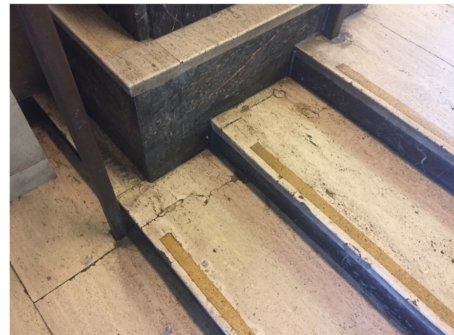
ALT-415 - Stone Floor Repairs Travertine stone is used within the entrance and borders the terrazzo across the main entrance area. Floor showing sign of damage. Cracking to be repaired with a matching resin by stone specialist, with hairline cracks and minor wear and tear are to remain in situ. Lose stone to be re-bed.
