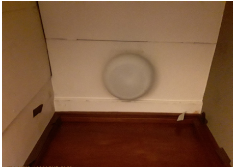
Existing lighting retained in concierge and Barrista with additional downlight to achieve required lux levels.
