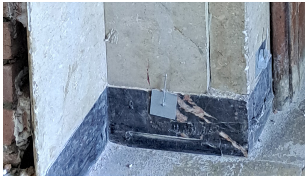
Skirting Ashburton Marble is used as a feature to skirting flush with the stone panelled walls. To be repaired as the method statement ALT-418.
