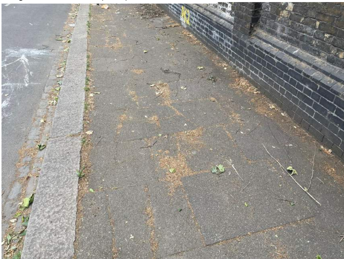
Image 42 - Parkview Rd (North) - Pavement condition
