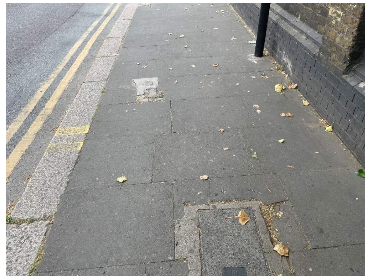
Image 31 - Parkview Rd (West) - Dowsett Rd Junction - Pavement condition & chamber
