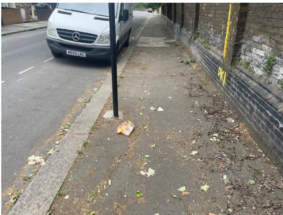
Image 46 - Parkview Rd (North) - Opposite 83 - Pavement condition
