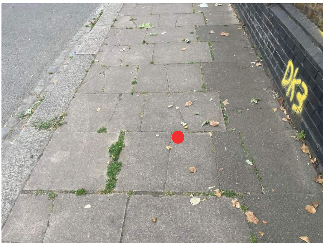
Image 37 - Parkview Rd (North) - pavement condition
