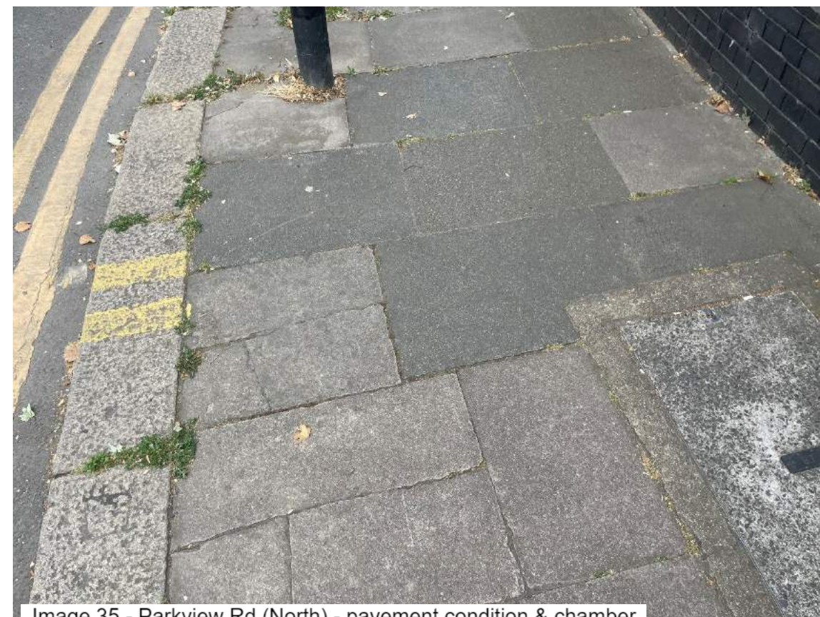
Image 35 - Parkview Rd (North) - pavement condition & chamber
