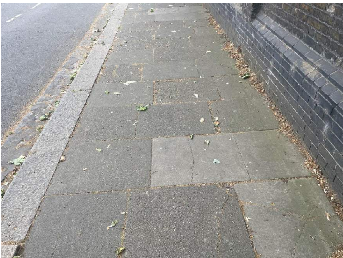
Image 53 - Parkview Rd (North) - pavement condition
