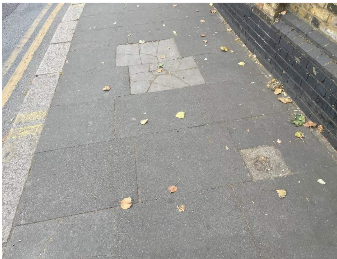
Image 29 - Parkview Rd (West) - Dowsett Rd Junction - Pavement condition
