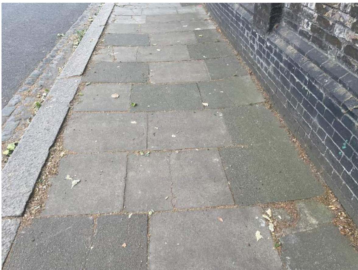
Image 52 - Parkview Rd (North) - pavement condition
