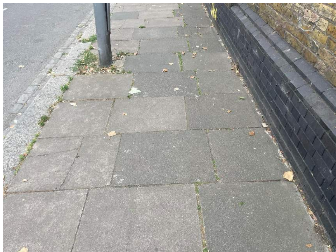
Image 34 - Parkview Rd (North) - pavement condition
