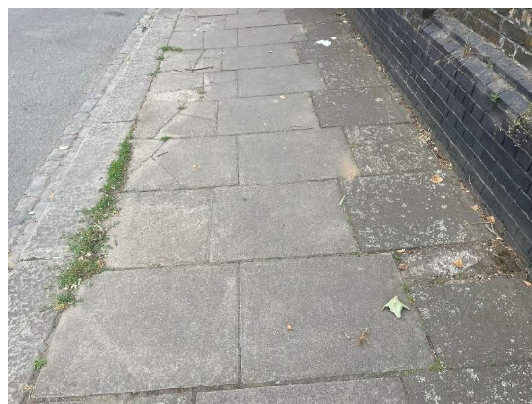
Image 40 - Parkview Rd (North) - pavement condition
