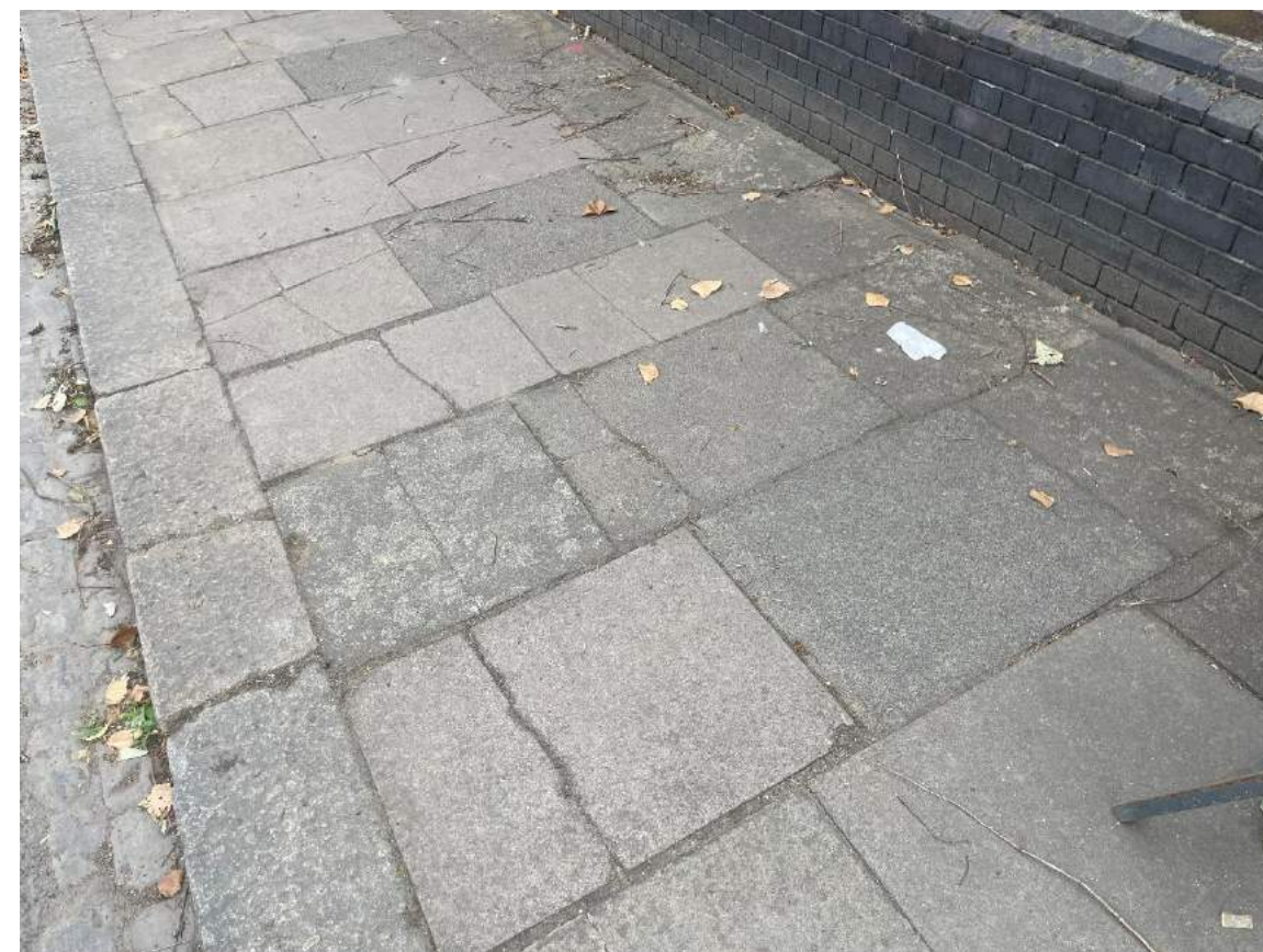
Image 43 - Parkview Rd (North) - Pavement condition
