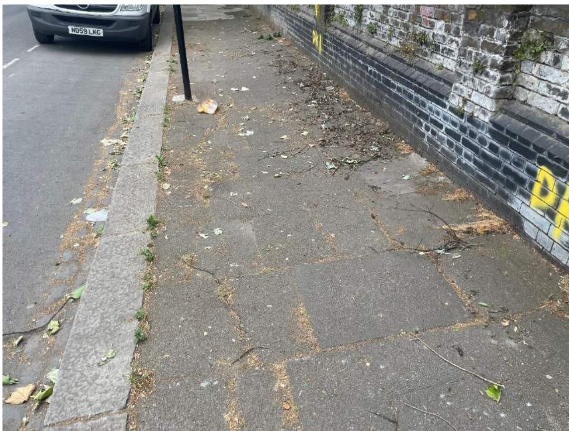
Image 45 - Parkview Rd (North) - Opposite 83 - Pavement condition
