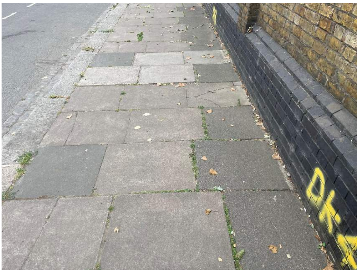
Image 41 - Parkview Rd (North) - Pavement condition
