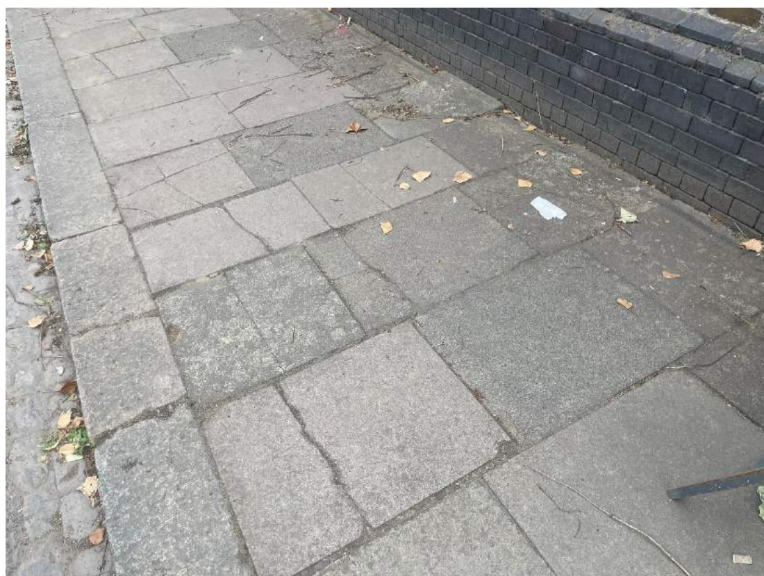
Image 38 - Parkview Rd (North) - pavement condition
