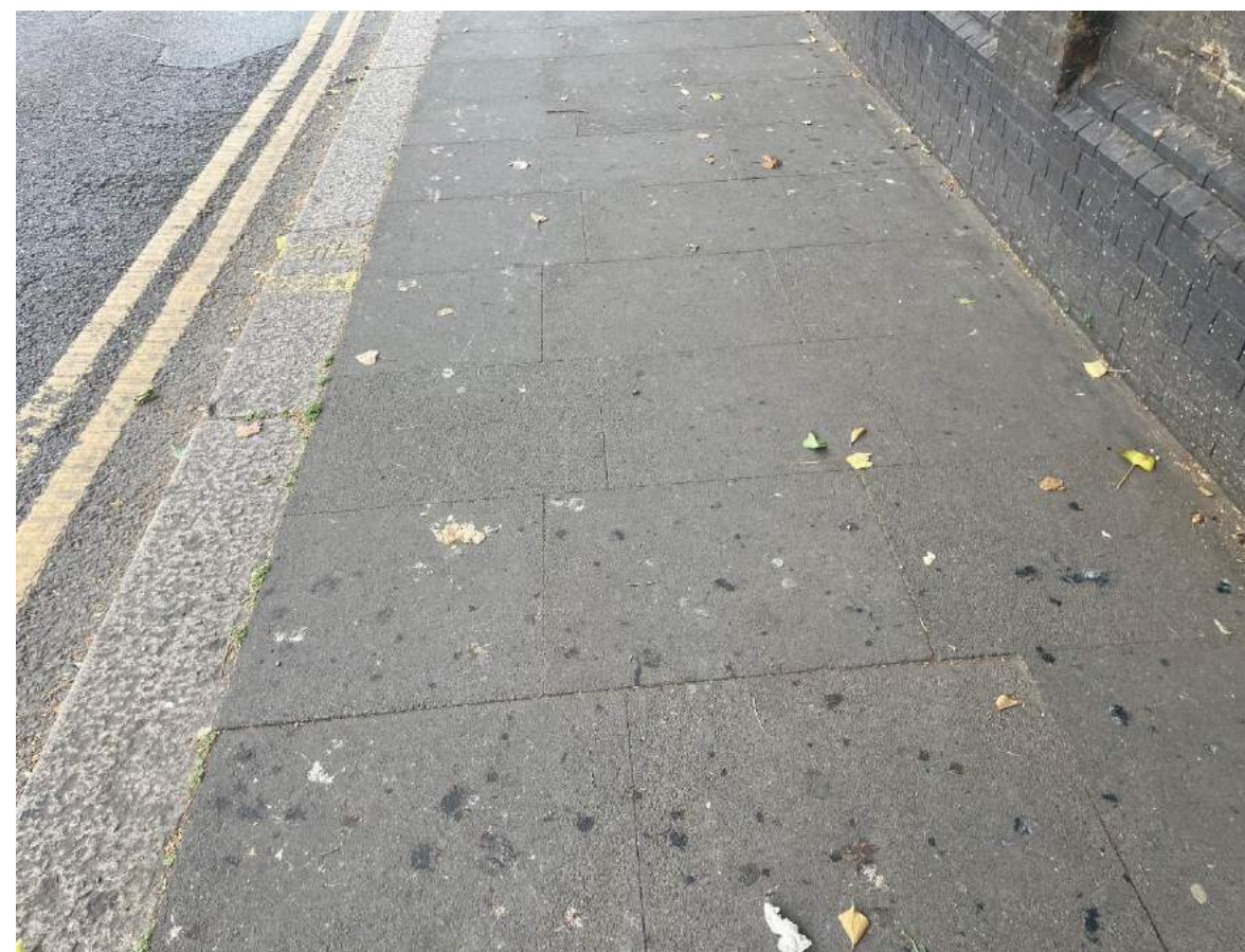
Image 32 - Parkview Rd (West) - Dowsett Rd Junction - Pavement condition
