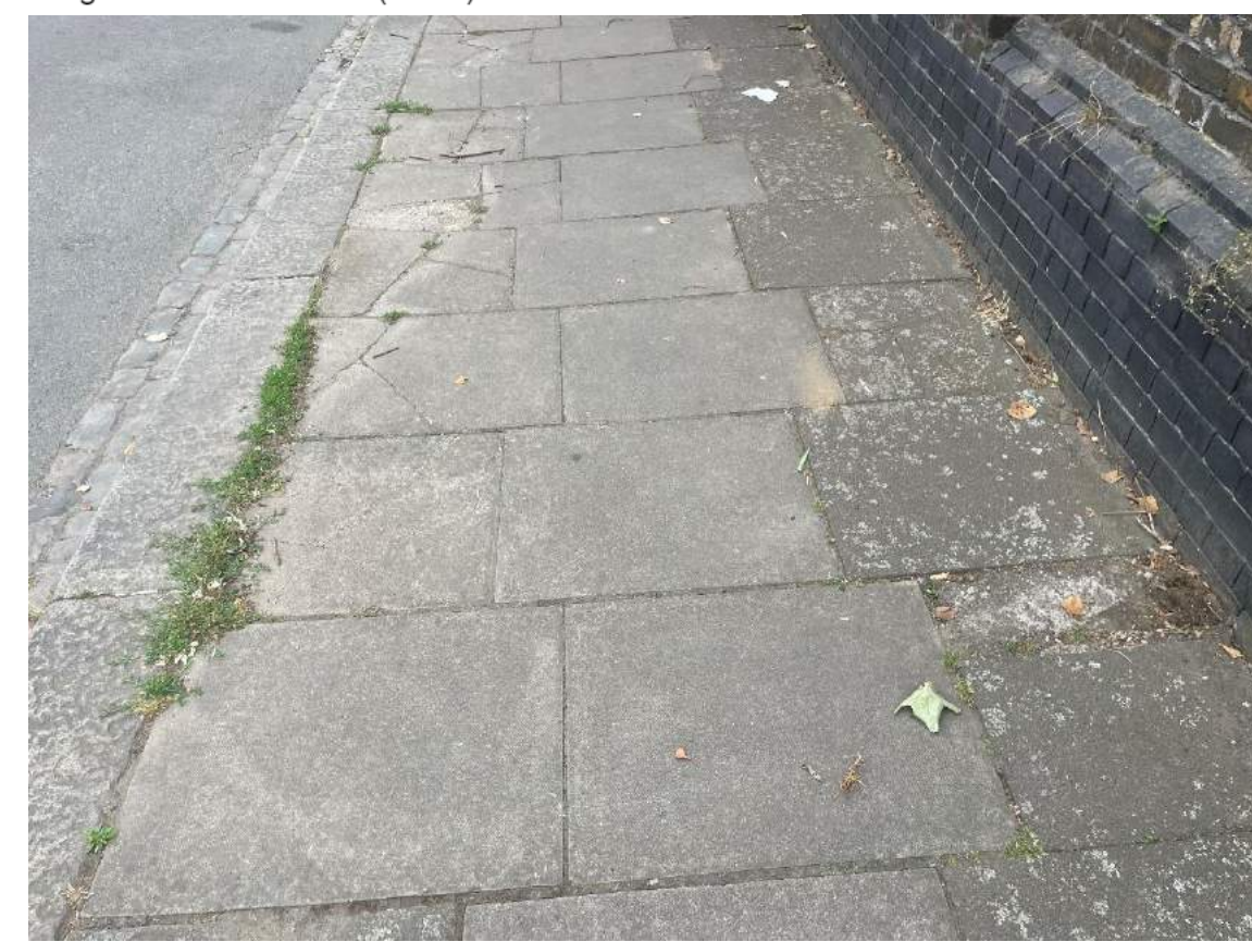
Image 44 - Parkview Rd (North) - Pavement condition
