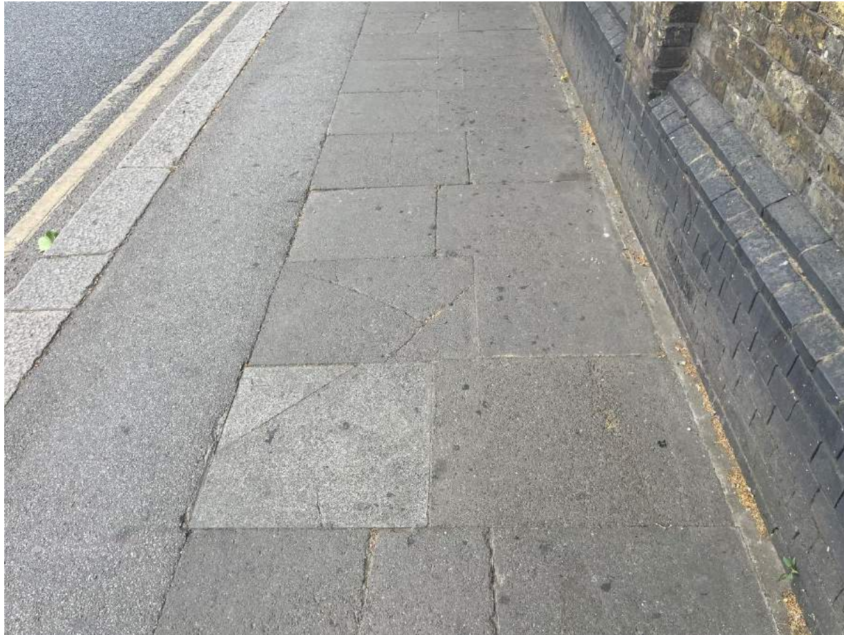
Image 17 - Parkview Rd (West) - Past Carew rd junction - pavement condition
