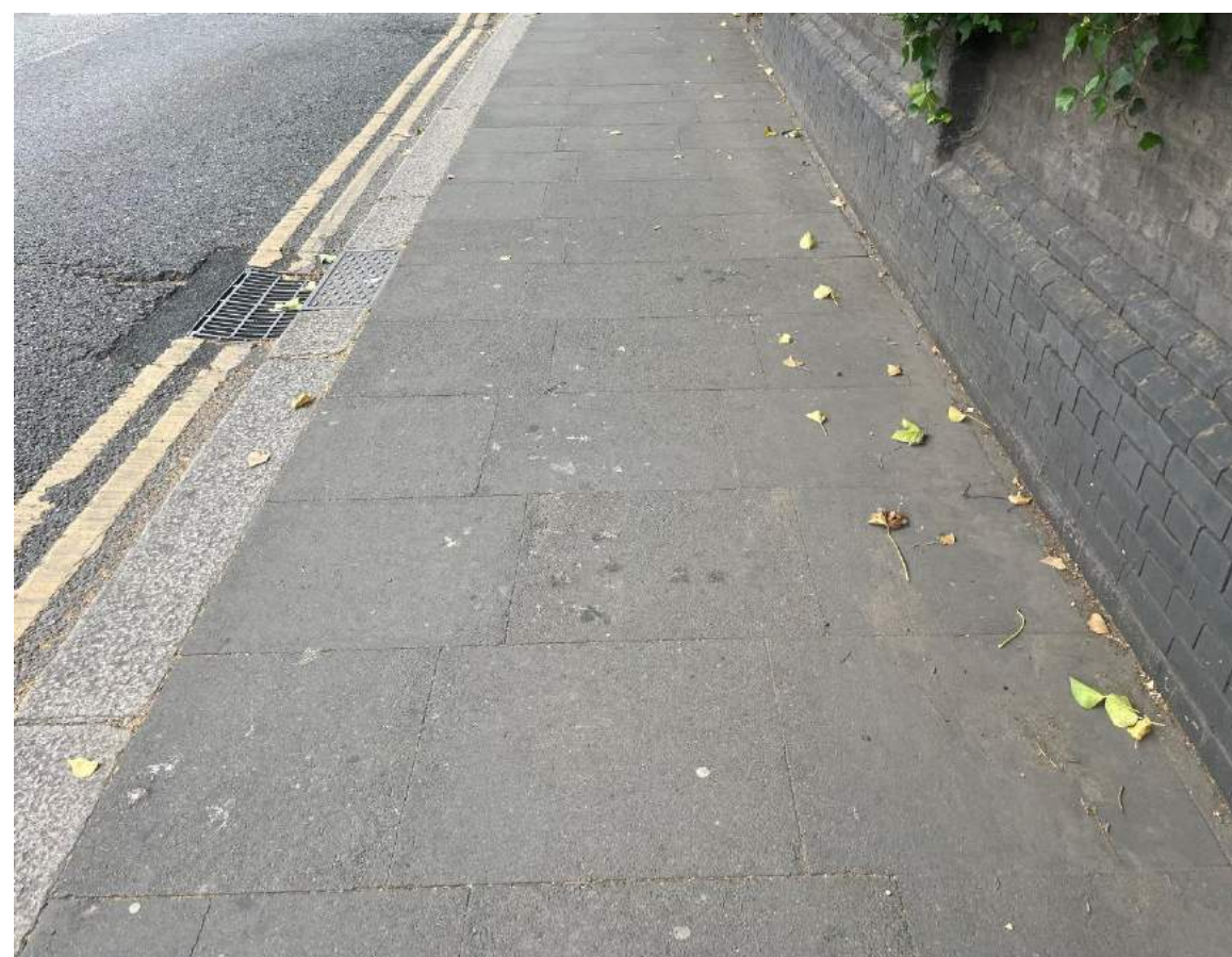
Image 30 - Parkview Rd (West) - Dowsett Rd Junction - Pavement condition
