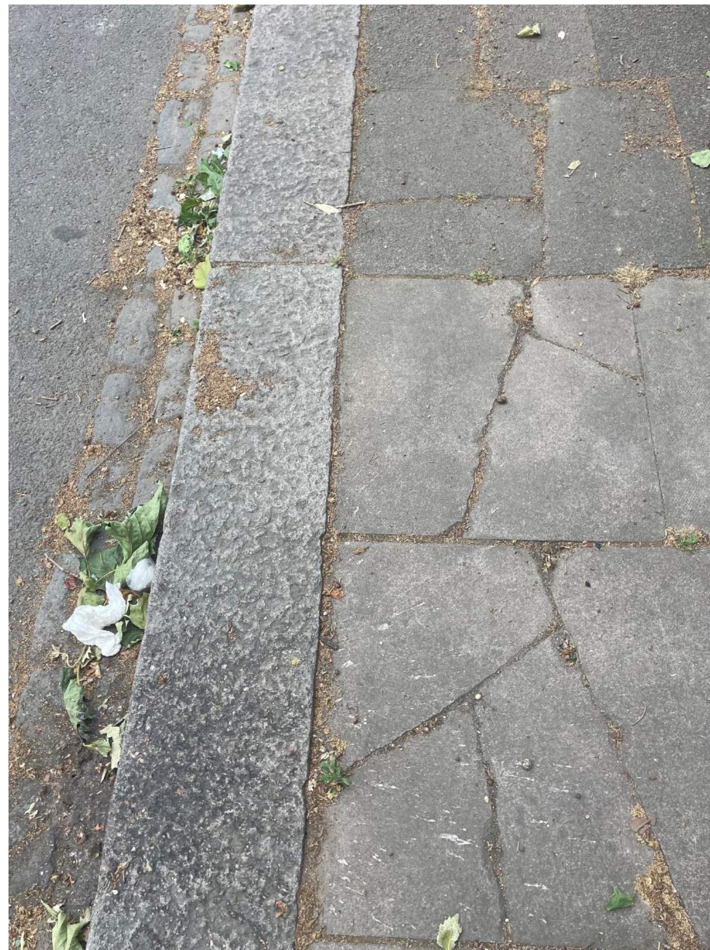
Image 47 - Parkview Rd (North) - Opposite 83 - Pavement condition
