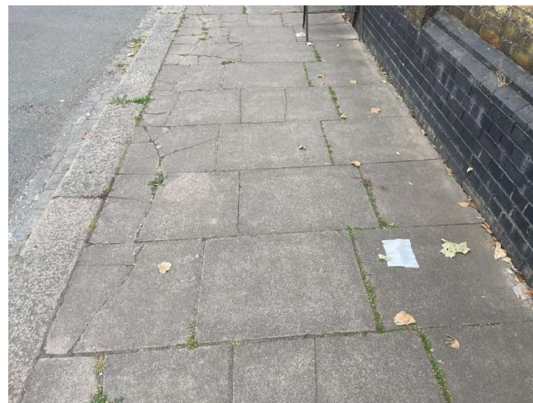
Image 39 - Parkview Rd (North) - pavement condition
