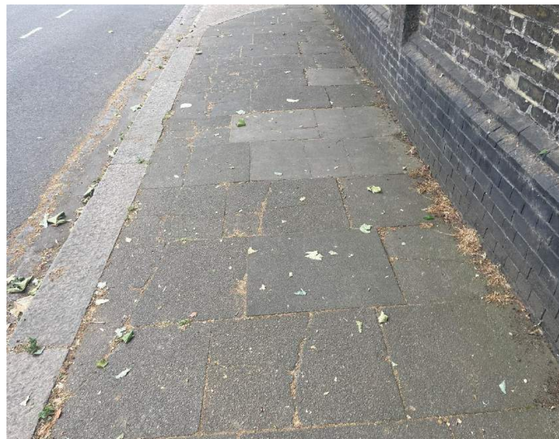
Image 55 - Parkview Rd (North) - pavement condition
