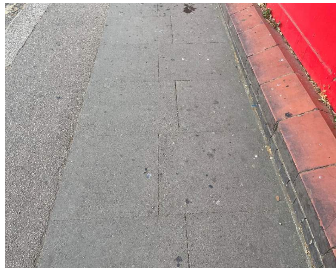
Image 28 - Parkview Rd (West) -Pavement condition
