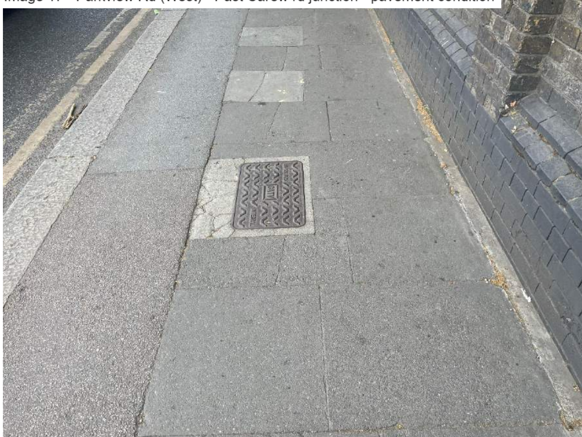
Image 18 - Parkview Rd (West) - Past Carew rd junction - pavement condition
